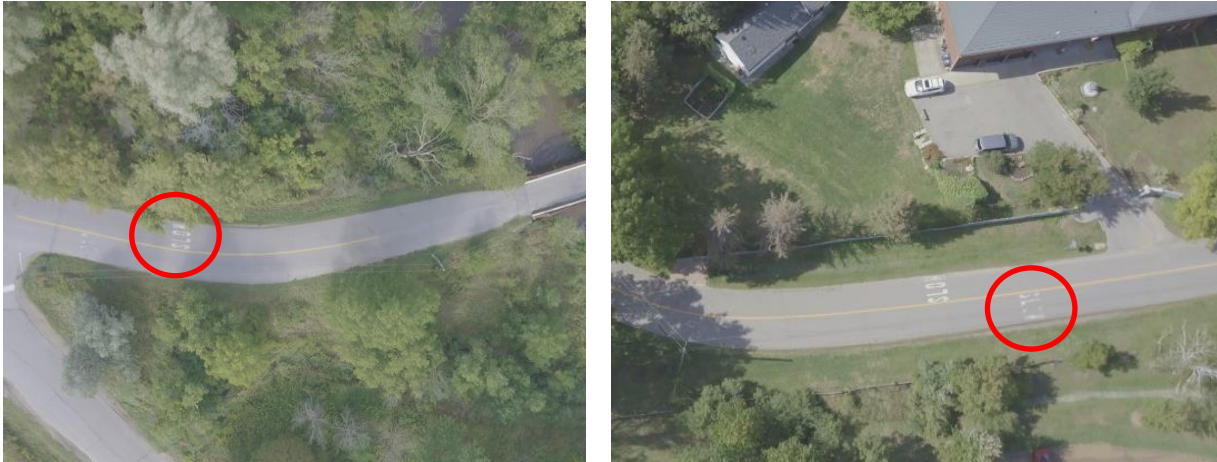
Figure 1: Clear Centreline and Faded "SLOW" Pavement Markings
