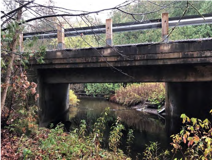
Plate 5: Northwest elevation of Bridge No. 1, concrete slab is clearly visible sandwiched between asphalt deck and concrete support beams.
