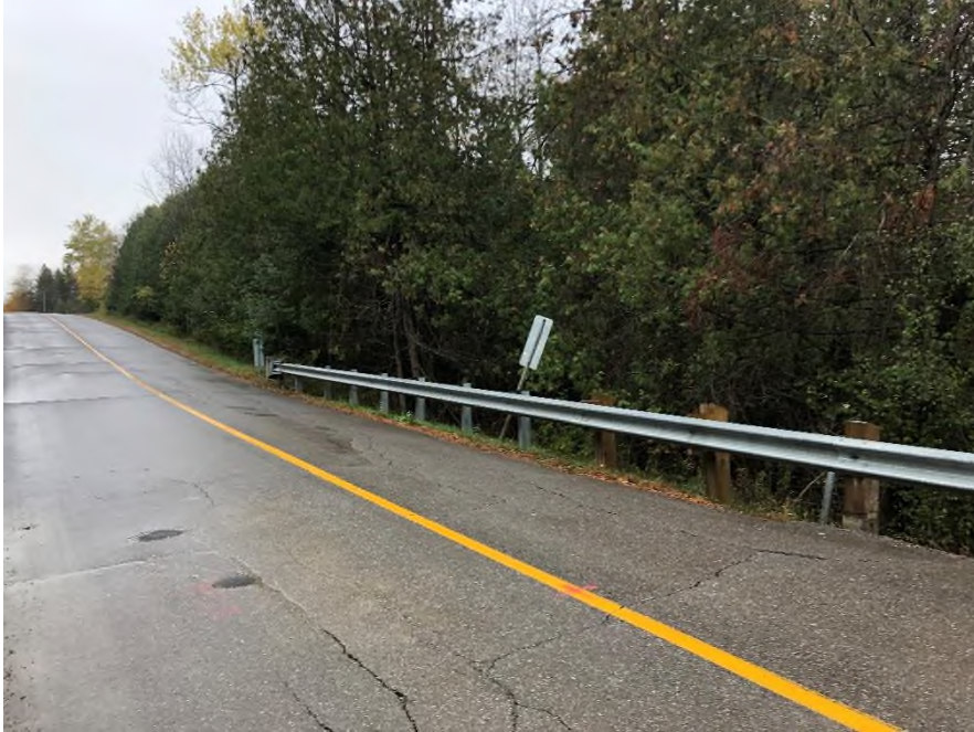
Plate 3: Bridge No. 1 flexbeam guiderails with galvanized steel posts lining the approach and wooden posts on the bridge.
