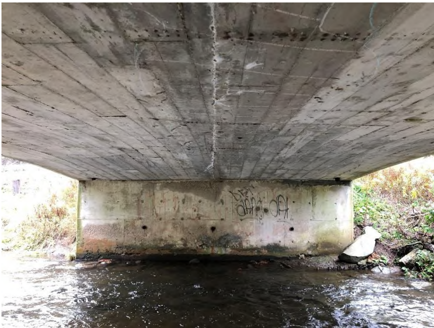
Plate 21: South abutment and underside of the superstructure. The seams indicating the location of formwork used to create the cast-in-place concrete is visible.
