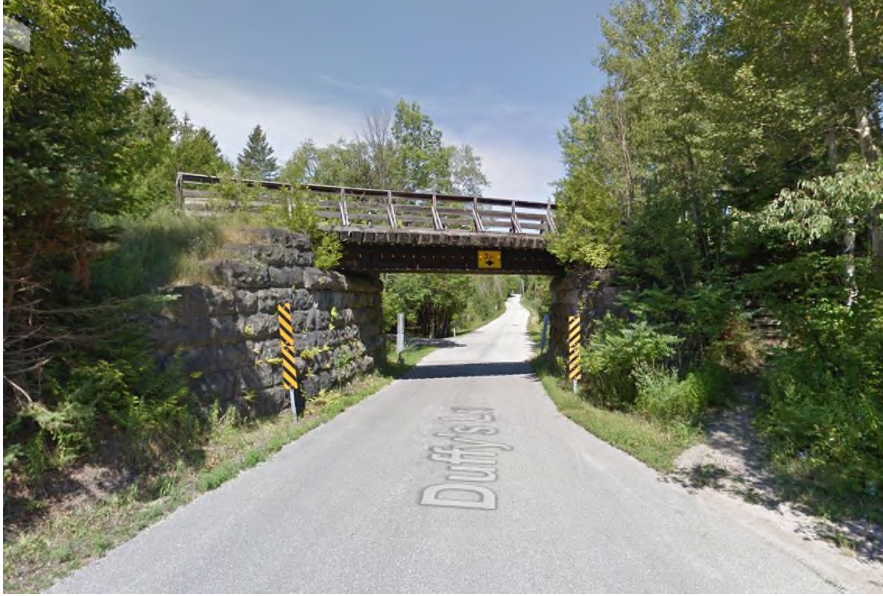
Plate 24: Caledon Trailway Bridge over Duffy's Lane, located approximately 180 m northwest of Bridge No. 2 (Google Maps, 2015)
