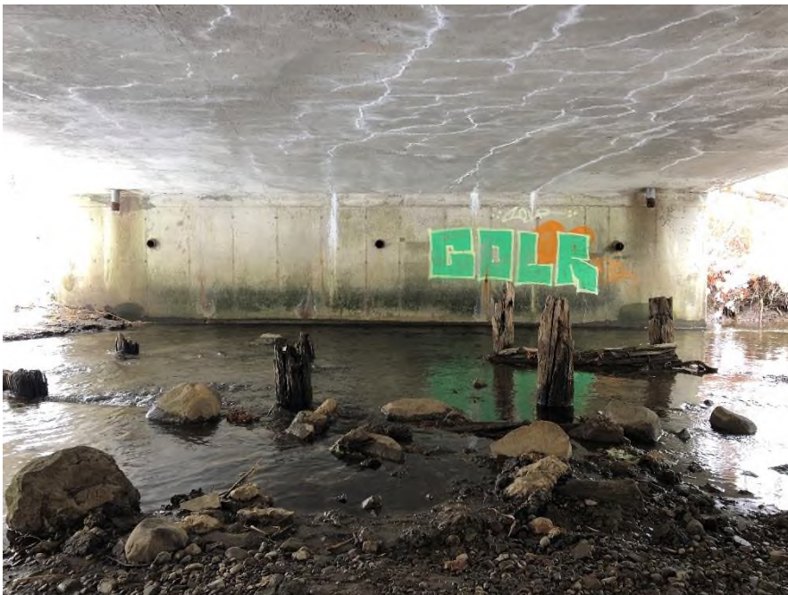
Plate 34: East abutment and underside of the superstructure. Wooden piles from a previous structure are visible within the waterway.
