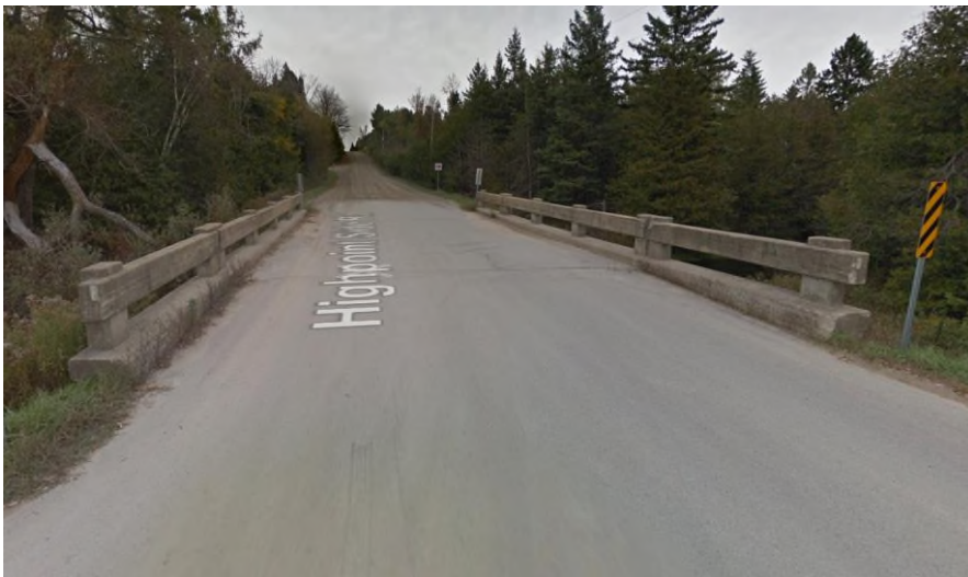
Plate 36: Highpoint Sideroad Bridge, located 0.02 km east of Shaws Creek Road (Google Earth 2016)
