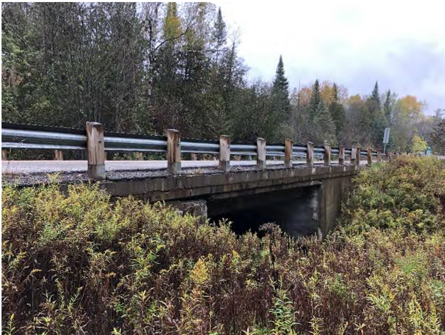
Plate 4: Oblique view of northwest elevation of Bridge No. 1, showing concrete slab and updated barrier system.
