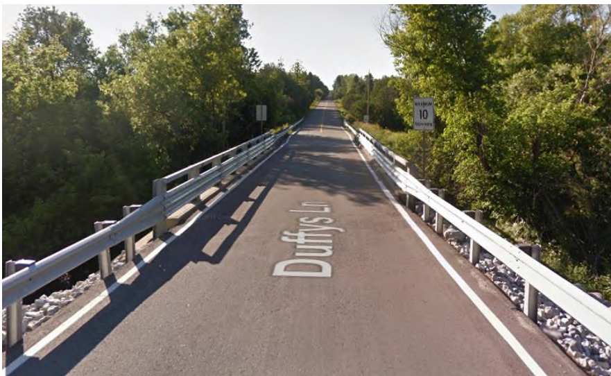
Plate 12: Duffy's Lane Bridge, constructed in 1950, located 1.7 km north of Castleberg Side Road (Google Street View 2016).
