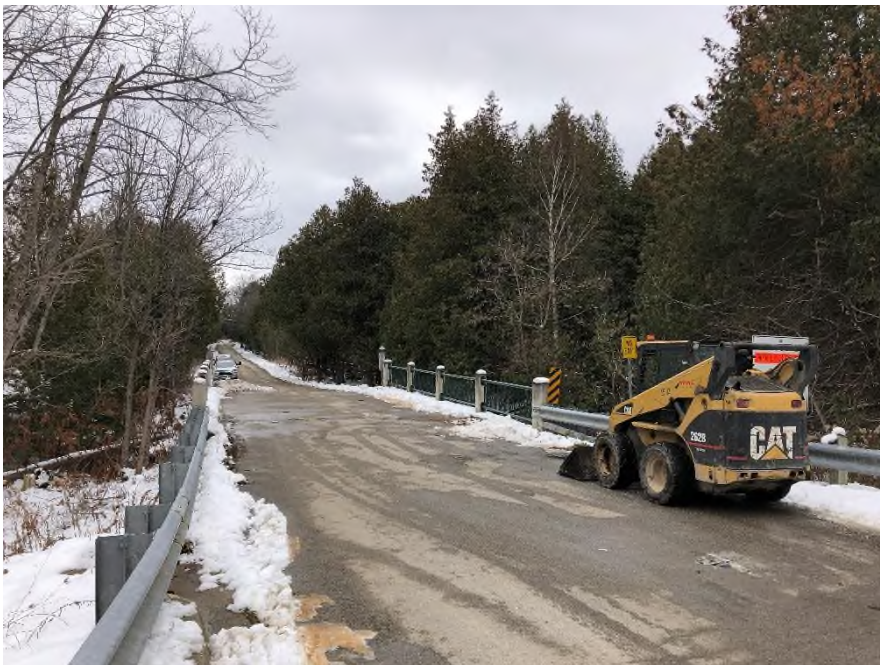
Plate 26: View southeast along western approach, from the intersection of Patterson Side Road and Duffy's Lane, towards Duffy's Lane Bridge.
