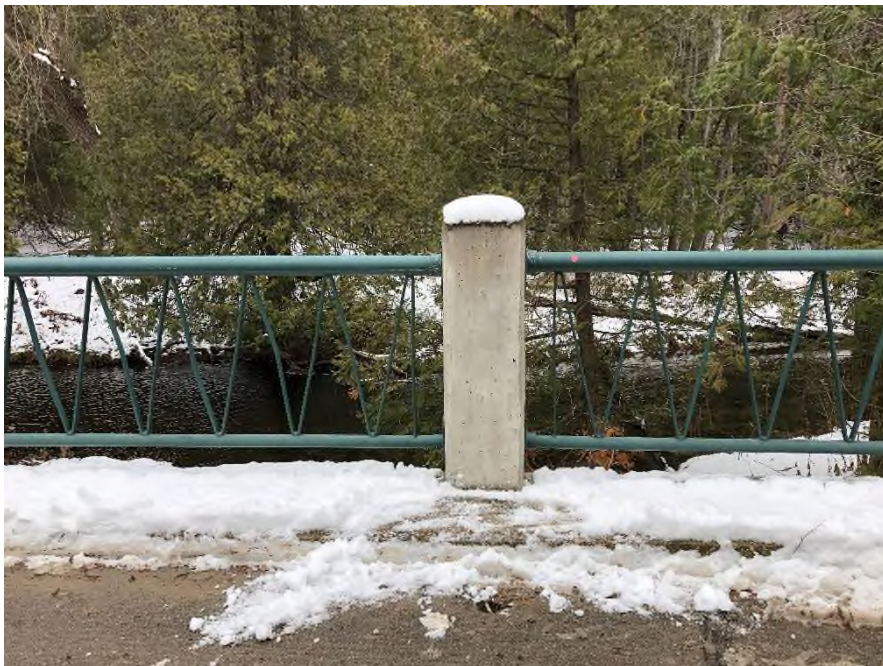
Plate 32: Detail of cement post and steel barrier system, rehabilitated in 2000 using recycled material and designs from original 1957 structure.
