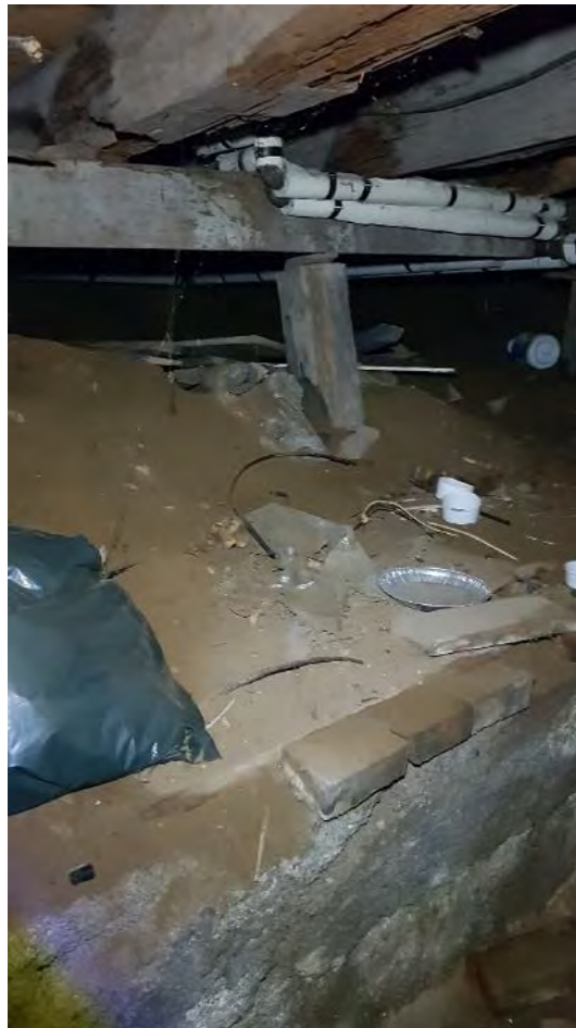
Figure 23: Dirt and concrete wall in the basement.
