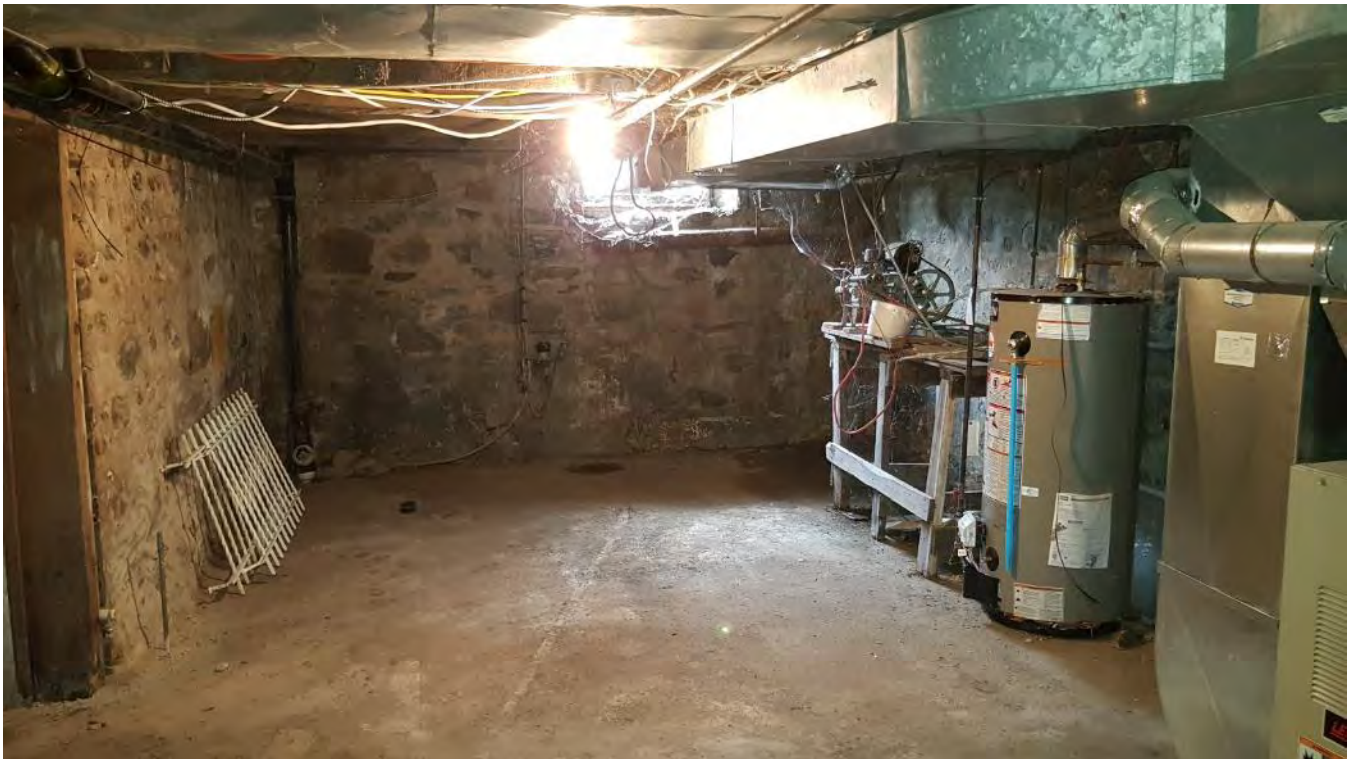
Figure 55: West basement room with furnace to the right.
