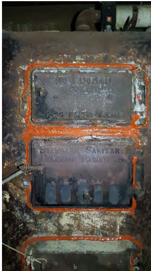
Figure 35: Dominion Radiator Ltd. boiler cover in the basement.
