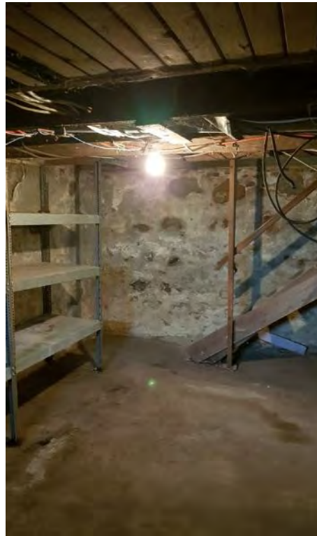
Figure 54: Basement with concrete flooring and fieldstone foundation which has been faced with concrete.
