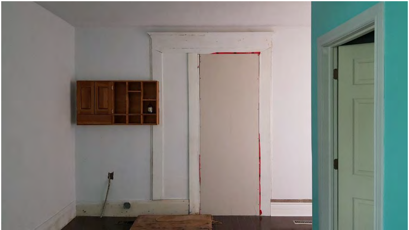
Figure 50: Large living space with boarded up entrance leading to the Northeast Extension.
