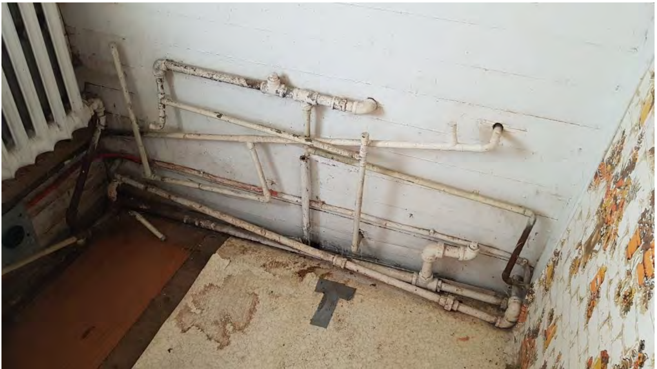
Figure 34: Pipe work in the kitchen.
