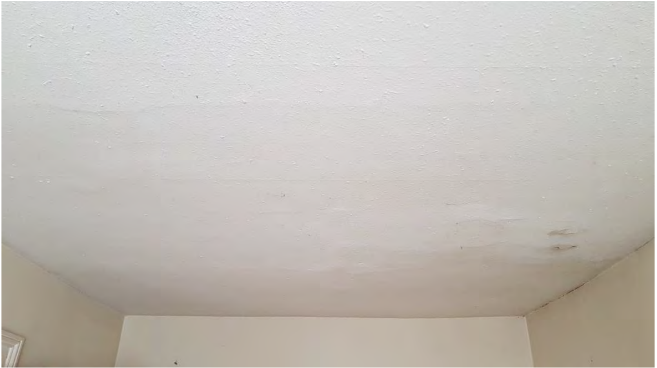
Figure 33: Evidence of water damage in living room ceiling.
