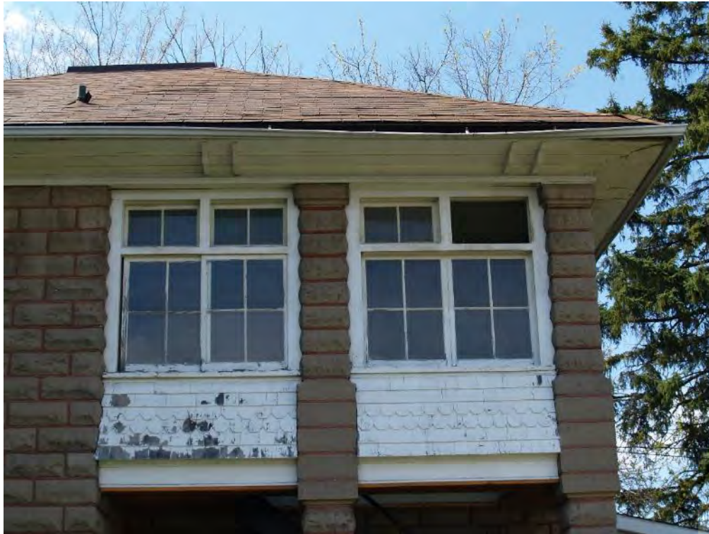
Figure 62: Broken gutter along the roofline and second-storey missing window pane.
