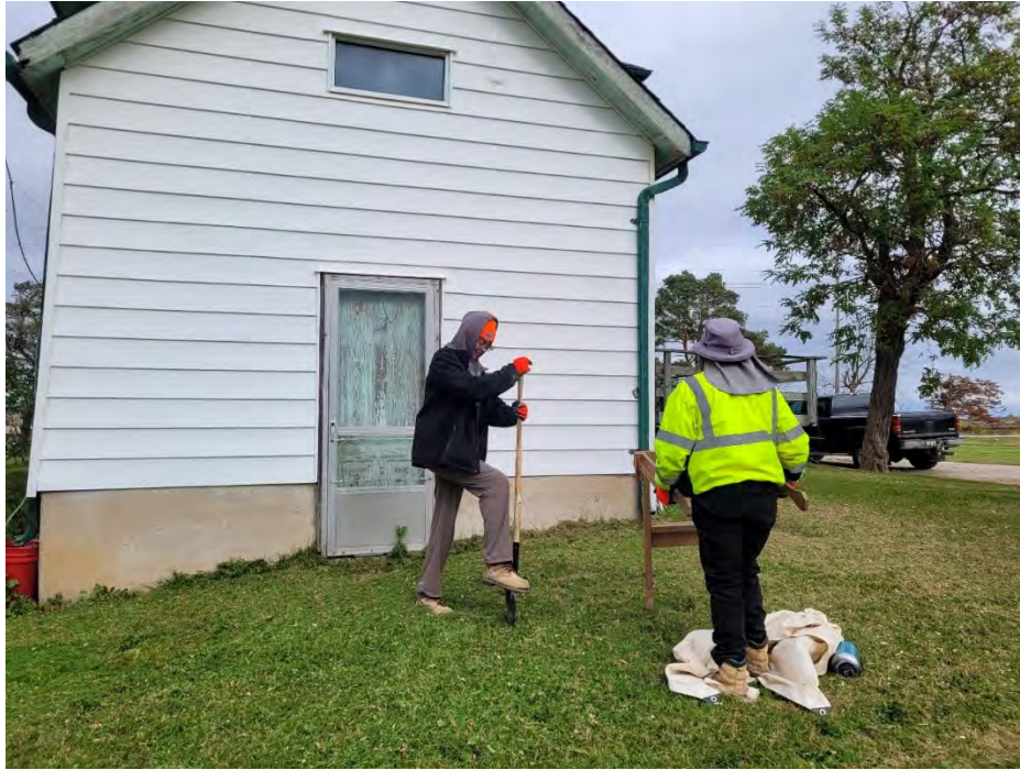
IMAGE 21: 12306 CHINGUACOUSY RD, TEST PITTING WITHIN 1M OF STRUCTURE AT 12306. VIEW FACING NORTH-EAST.
