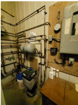
Picture 47: View of the electrical panel in the Maintenance Barn.
