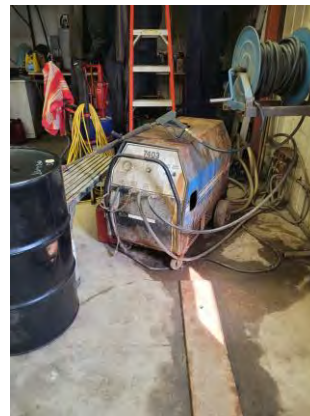
Picture 46: View of the generator in the Maintenance Barn.
