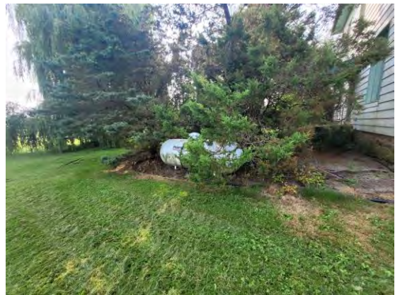
Picture 10: View of the house's propane tank, north of the house.
