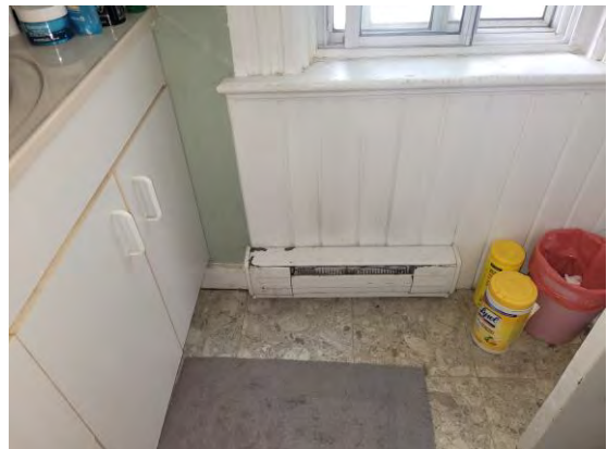
Picture 12: View of the baseboard heater in the bathroom, facing south.
