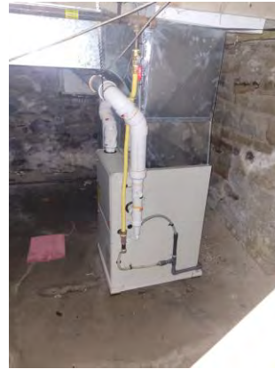
Picture 14: View of the furnace in the basement.
