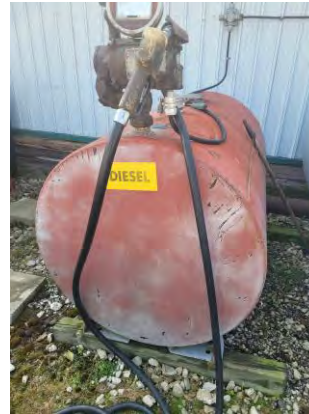
Picture 32: View of the 2 nd active diesel fuel tank beside Storage Barn 2.
