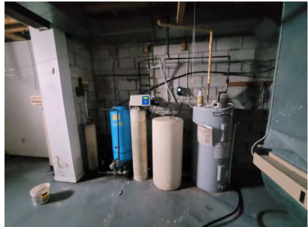
Picture 8: View of the water system in the basement.
