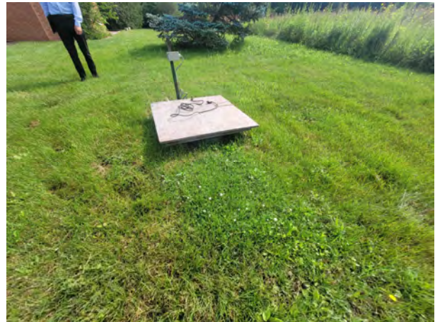
Picture 14: View of the septic system to the southeast of the house.
