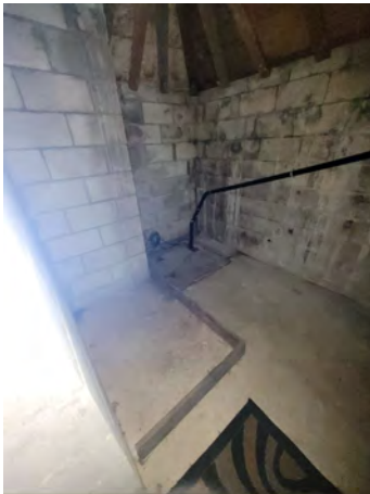
Picture 9: View of the sump pump in the basement.
