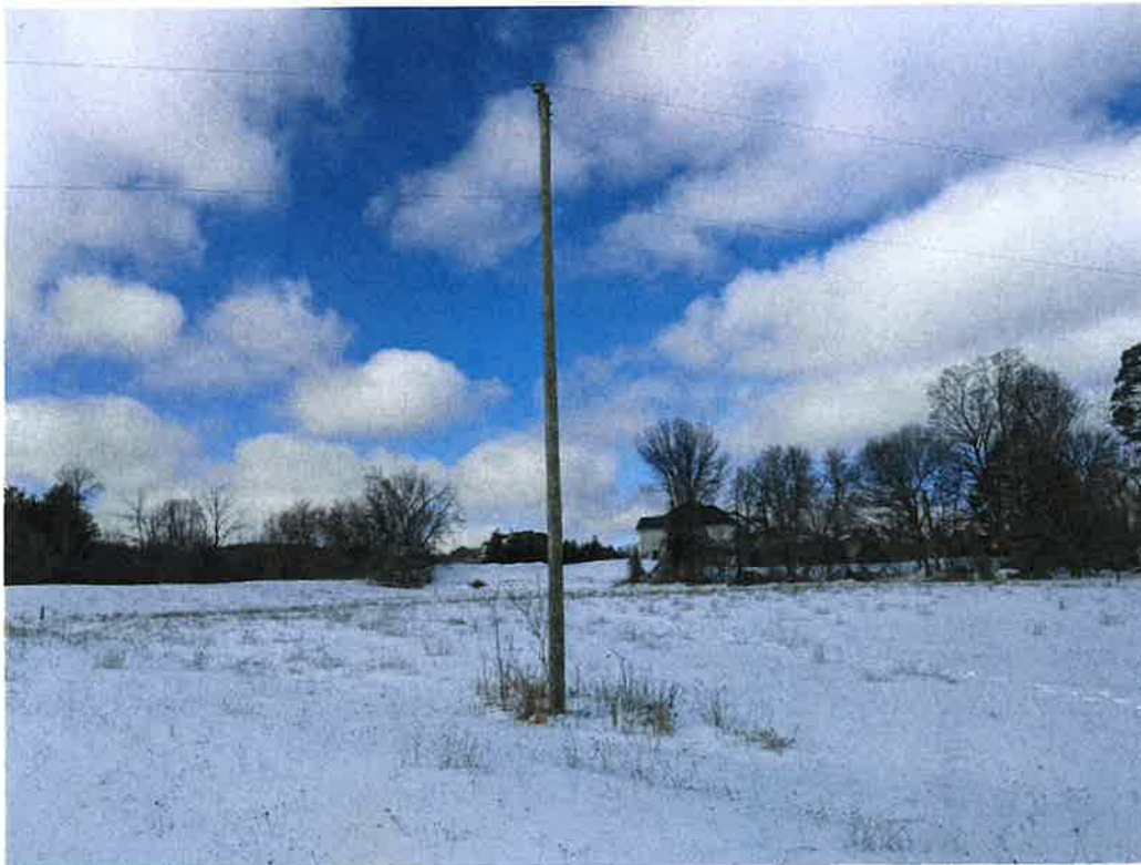
General view of existing hydro pole on subject site with overhead lines visible (looking west)
