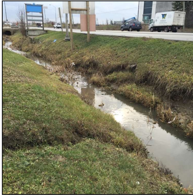
Photograph 1. Channel along Regional Road 50 showing slumping of the slopes and erosion gullies
