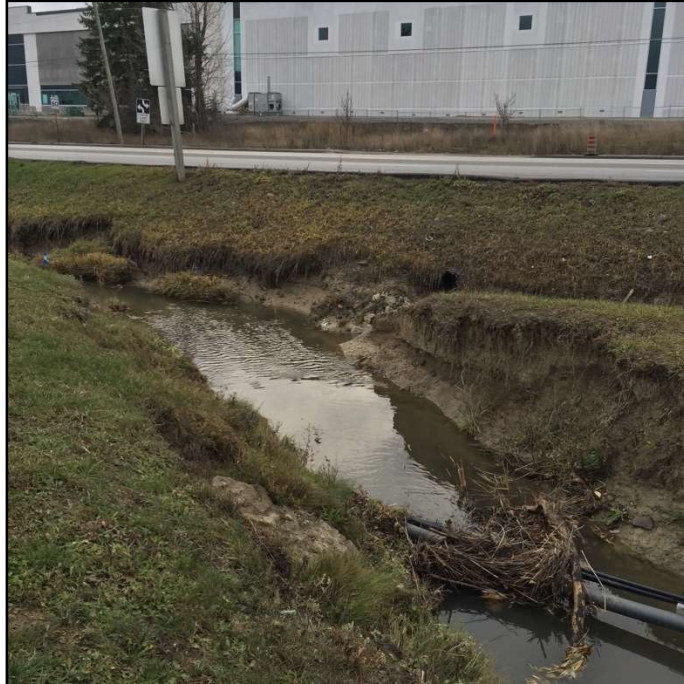
Photograph 4. Exposed service cables/pipes at the tributary as it joins the drainage ditch along Regional Road 50
