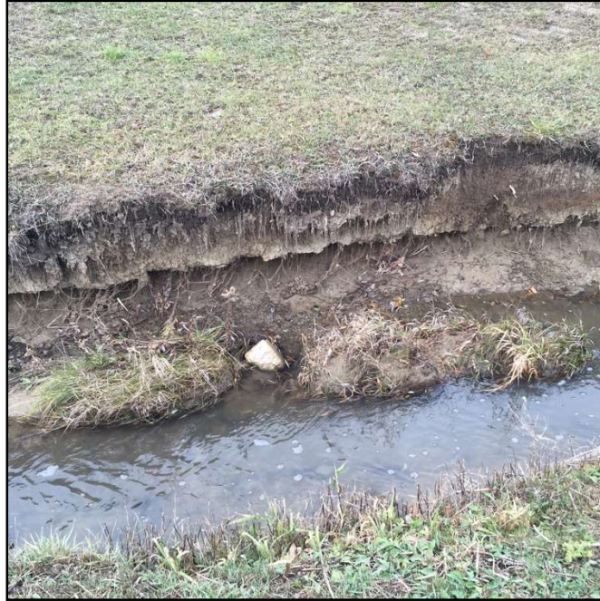
Photograph 2. Typical slope slumping and erosion observed along the entire channel
