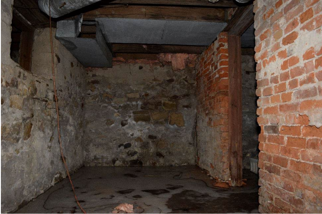
Figure 78: Central room in south half of basement, facing south, wall in centre of image would be under front door
