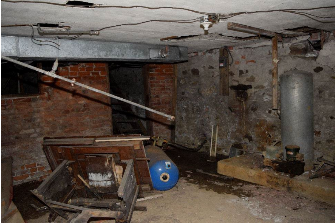
Figure 75: Basement, main foundation is of field stone with internal partitions of red brick
