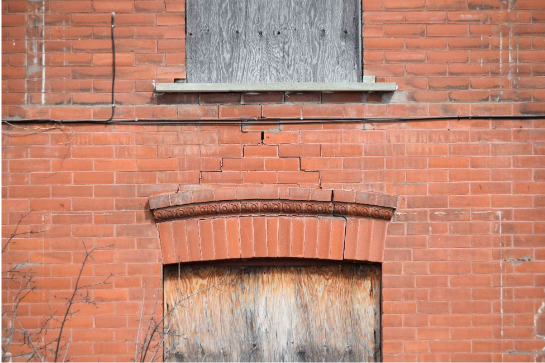
Figure 31: Example of typical brick failure associated with structural openings
