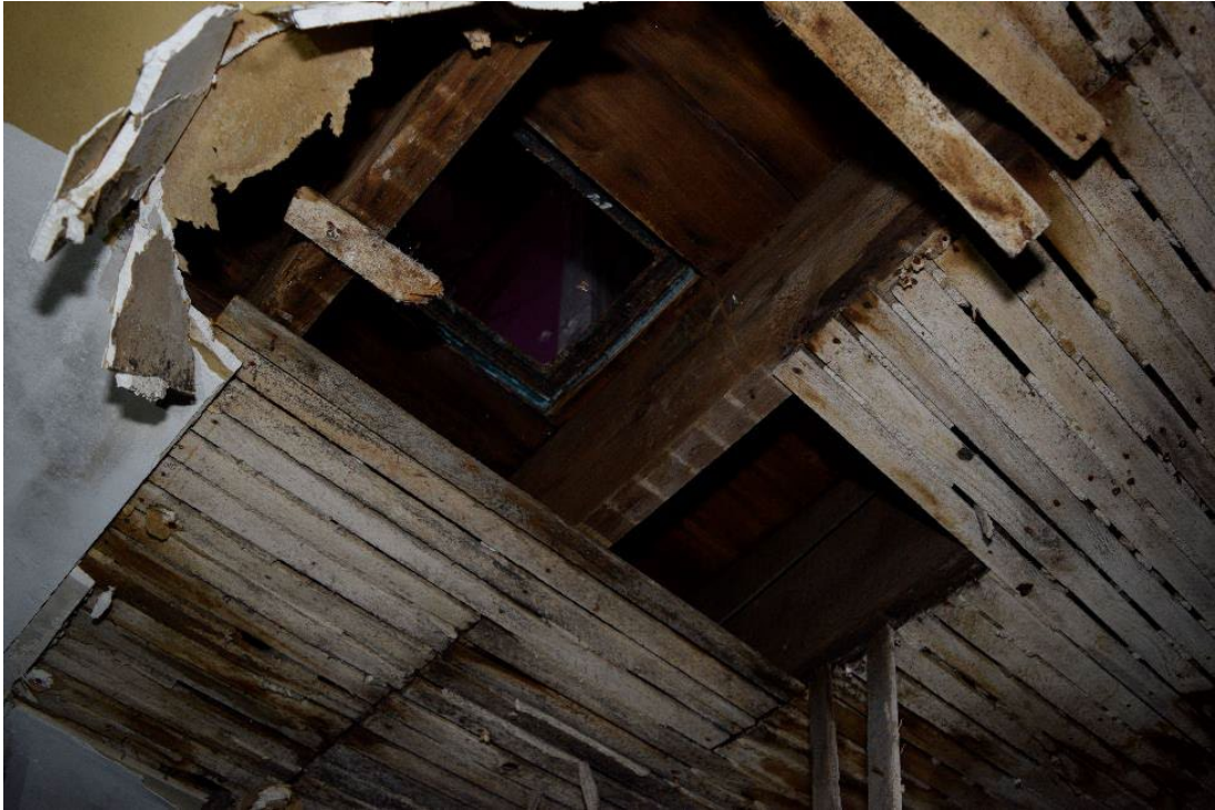
Figure 81: Example of extensive internal damage resulting from water and vandals
