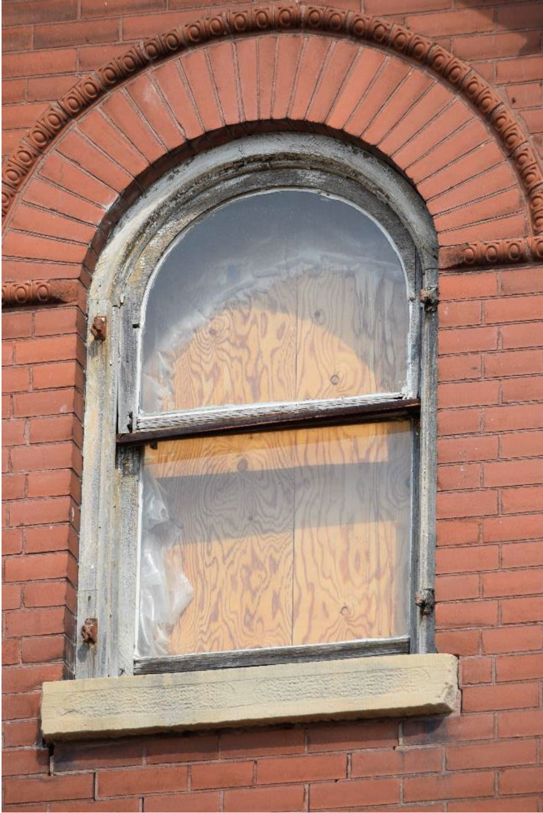
Figure 28: Round-headed single hung sash window in centre dormer, note original shutter installation hardware
