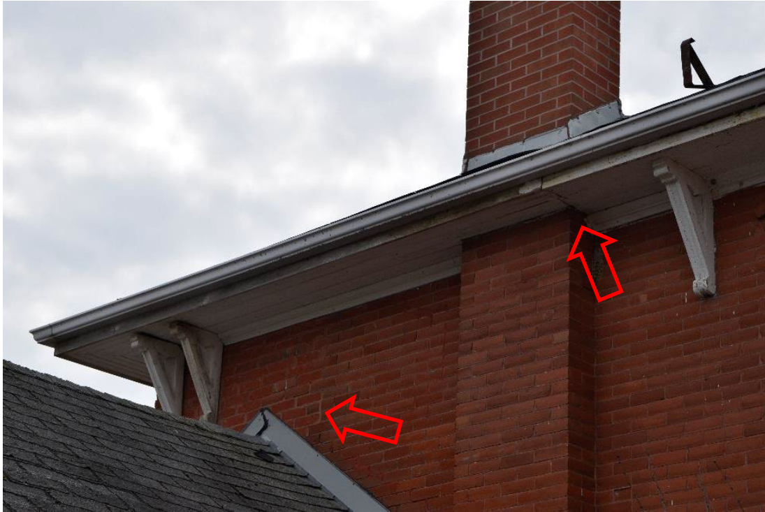
Figure 37: Damage in northeast corner of structure's north face, red arrows indicate transition between original material and replacement in both brick and soffit
