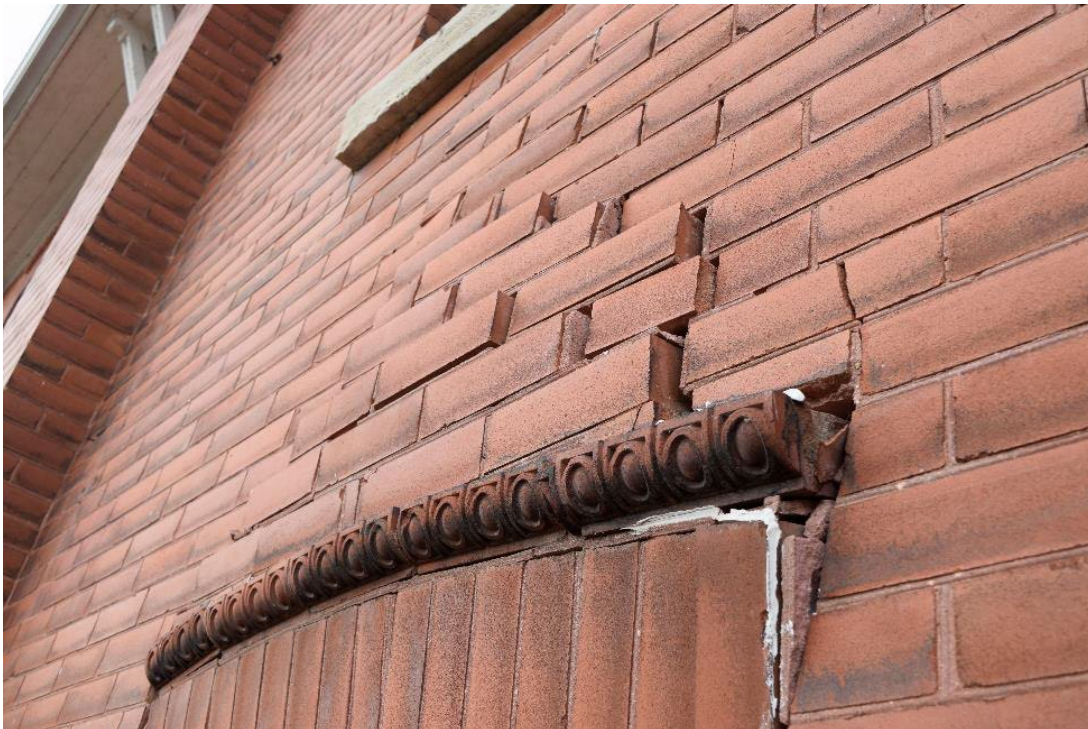
Figure 34: Close up of damage depicted in Figure 33
