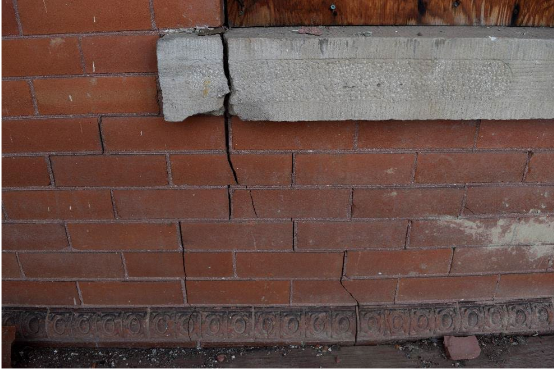
Figure 39: Stress crack in stone lug sill and brick work, east wall
