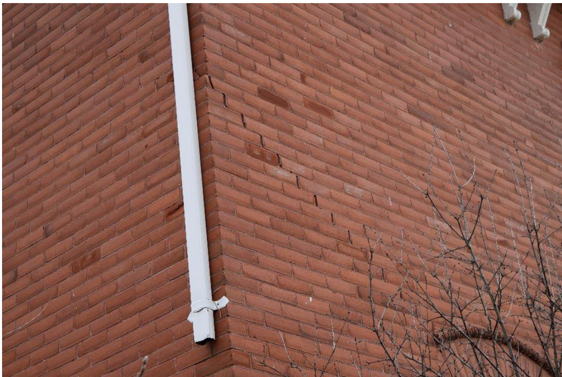
Figure 38: Stress crack in northwest corner indicative of foundation settlement
