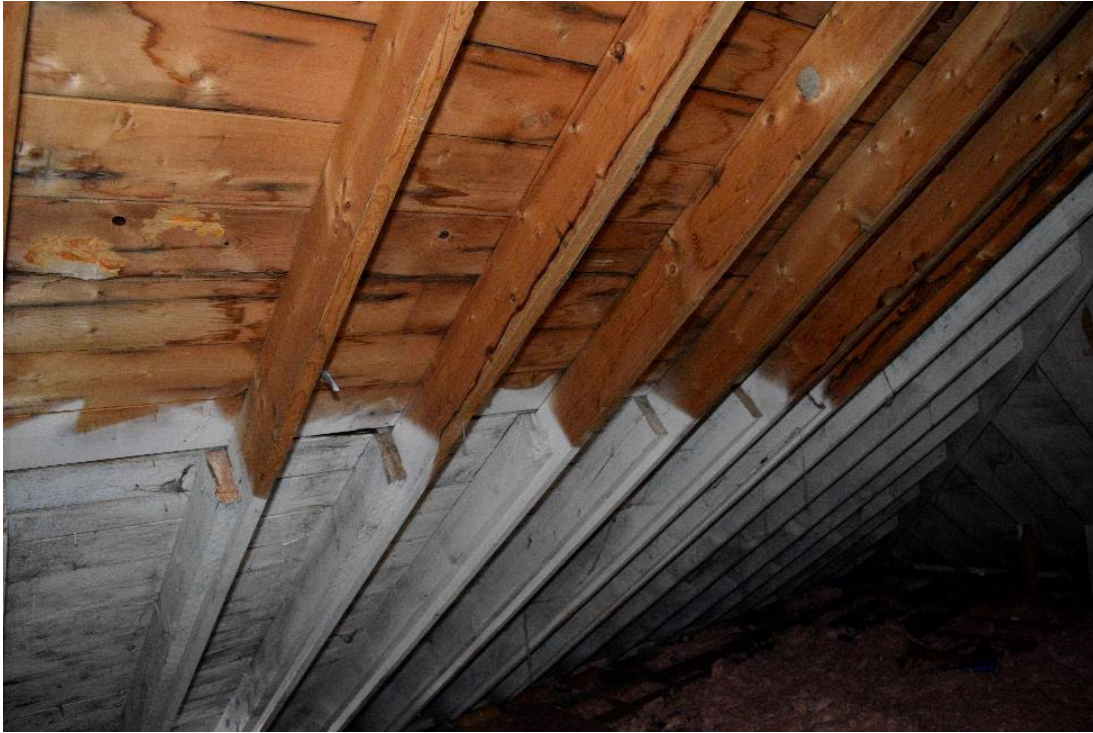
Figure 72: Evidence for extensive roof repair on west side of structure. The white line illustrates the connection between original framing and modern 2x6 rafters
