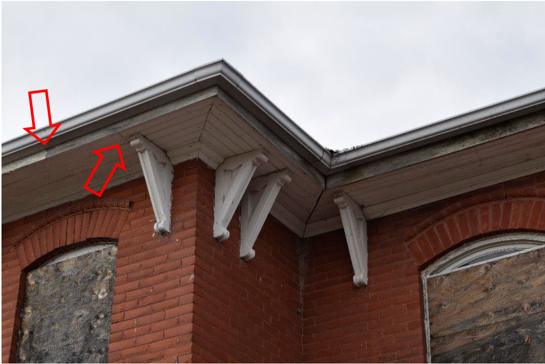
Figure 36: Close up of replacement fascia, soffit, and brackets, red arrows indicate seam between original and replacement materials
