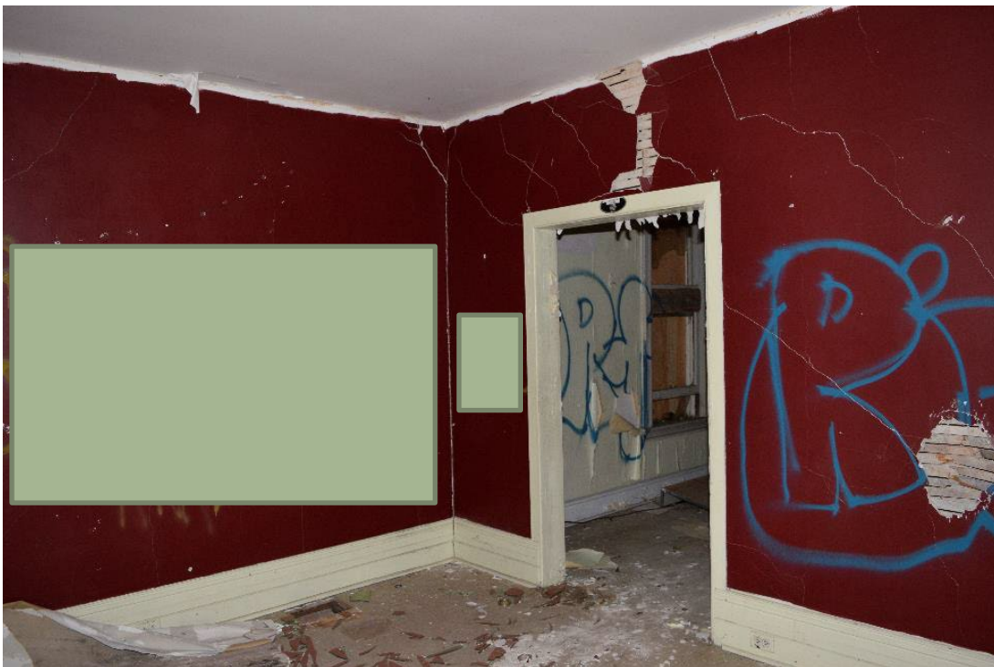
Figure 49: Later door added to north wall of southwest room first floor, note trim differences, vulgar graffiti digitally covered
