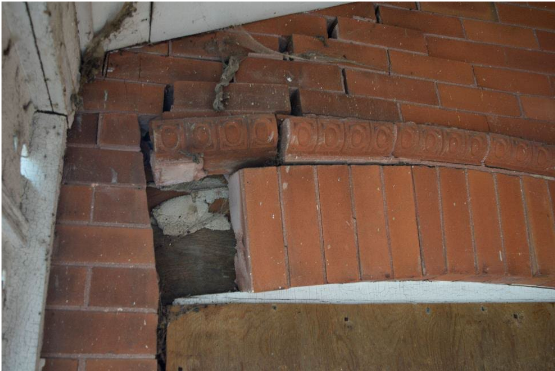
Figure 32: Closeup of typical failure of brick cladding
