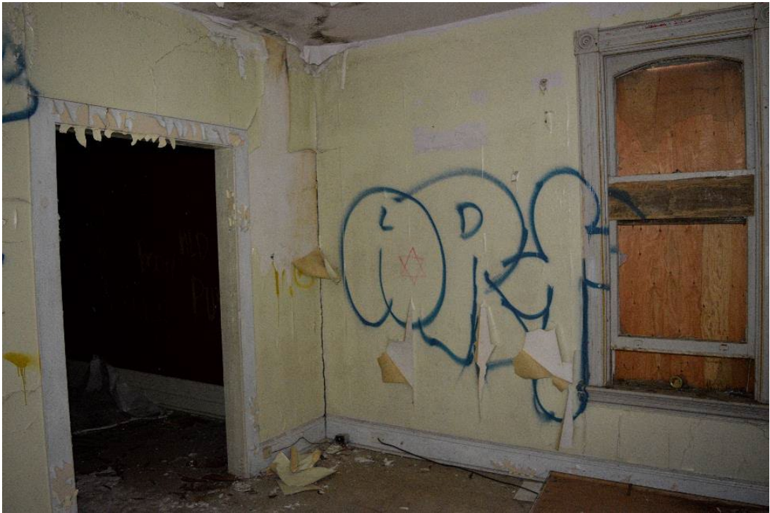
Figure 51: Later door added to south wall of central room on west side of structure
