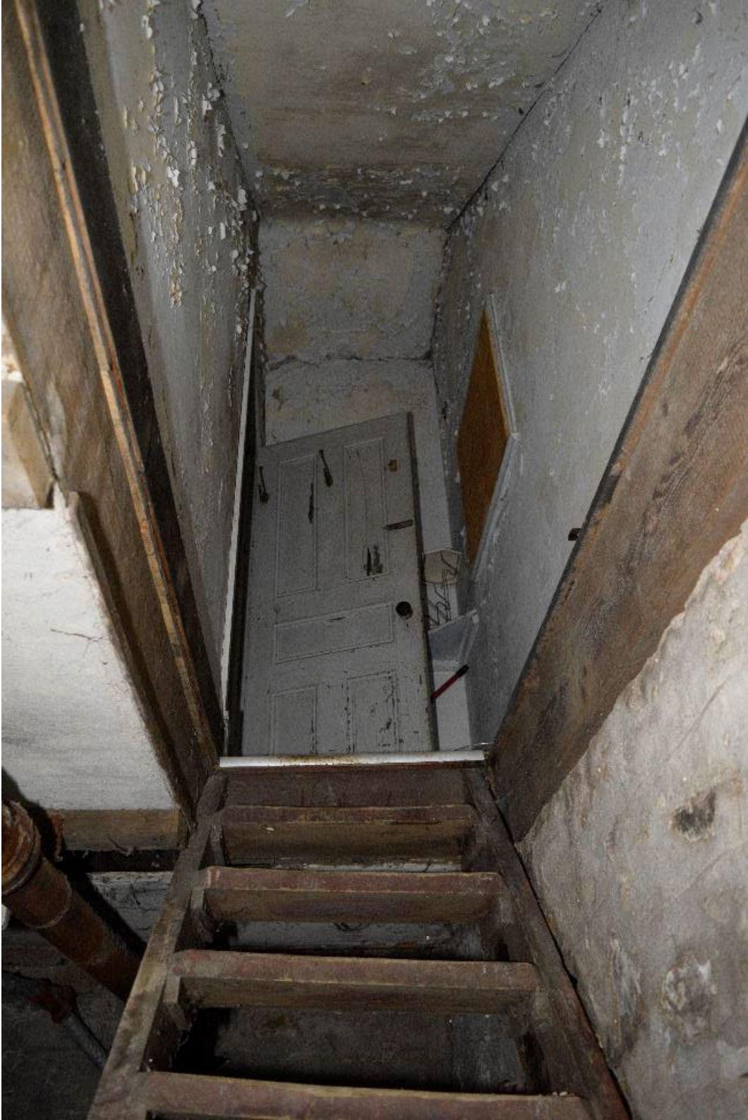
Figure 80: Internal stairs to basement, locate in northwest corner of structure, facing west
