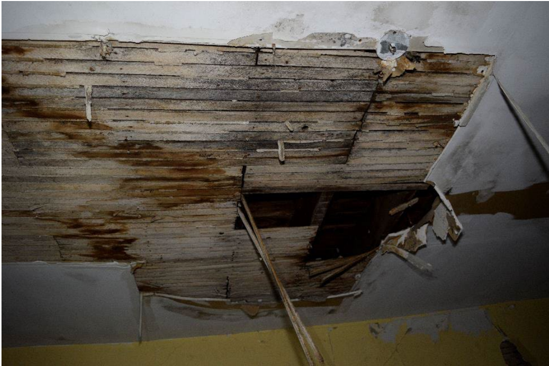
Figure 82: Drywall has been fastened over original lath; lath remains in most areas, but plaster has been removed thought house
