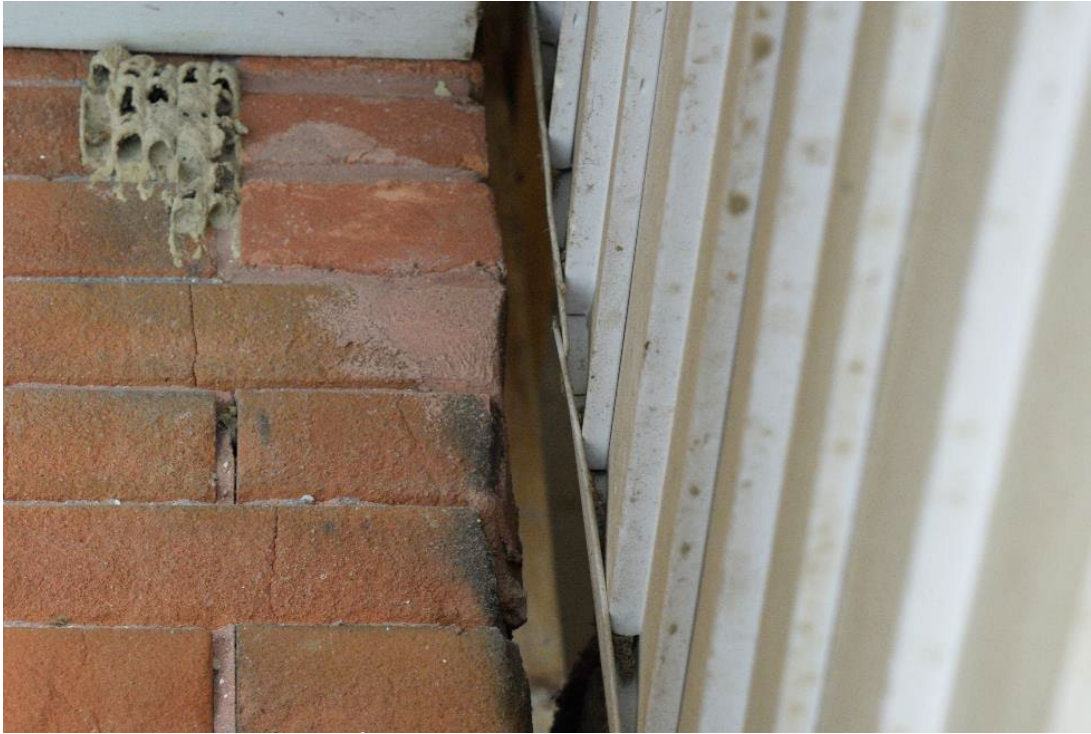
Figure 40: Large separation between modern addition and north wall of original structure, gap extends around structure and provides sight line to interior of structure
