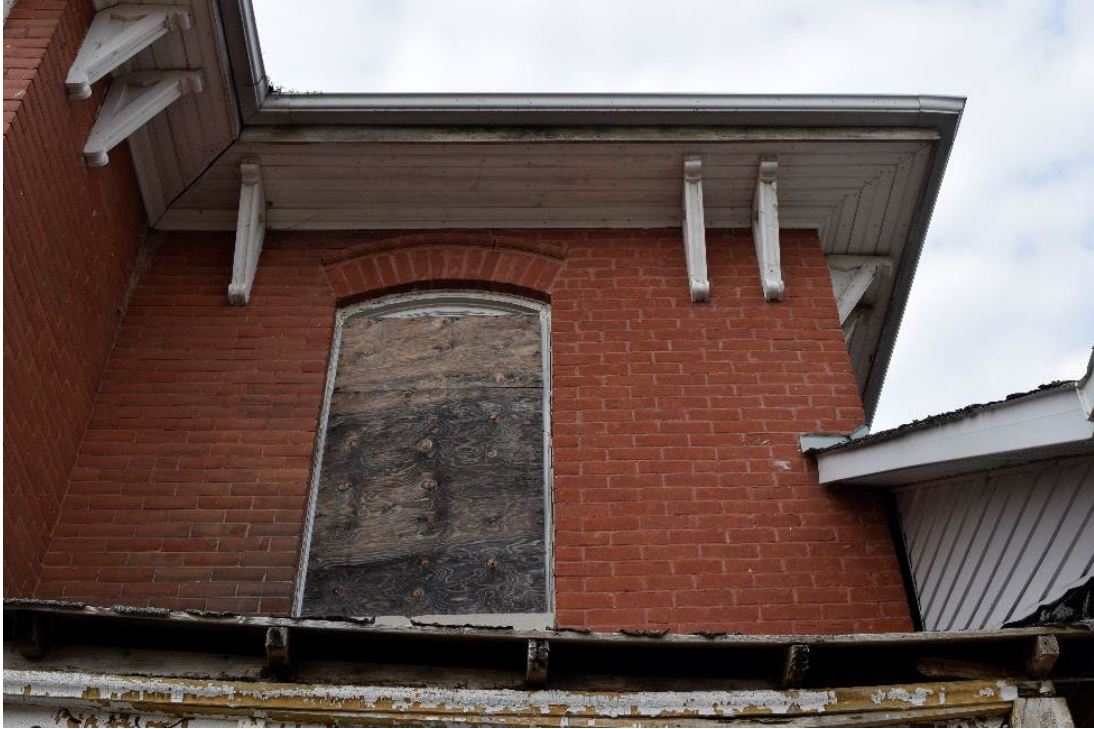
Figure 35: Past failure of the brick finish and replacement of the eaves, soffit and brackets on northwest corner, note mortar difference between right and left of image
