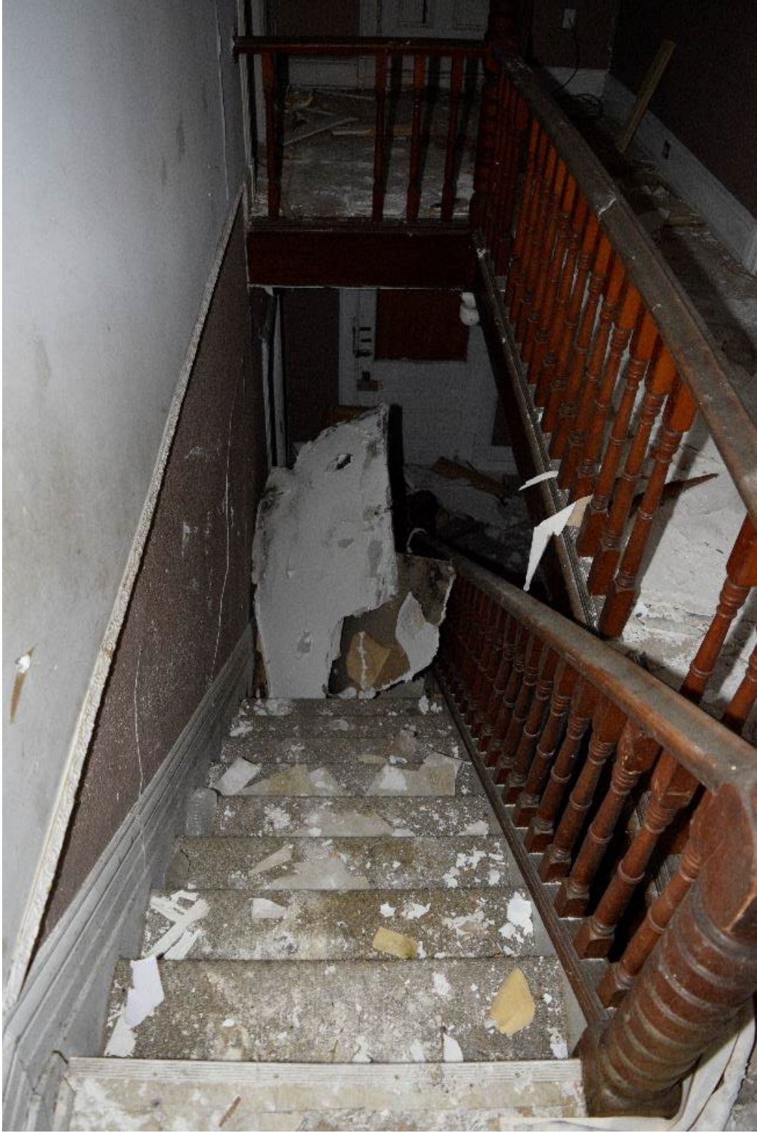
Figure 68: Stairwell, vandals have thrown cast iron tub through the stairs, currently covered in drywall, facing south
