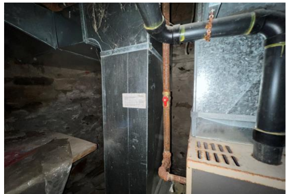
Picture 30: View of the manufacturing information of the furnace located in the basement of Old Heritage home, facing northeast.
