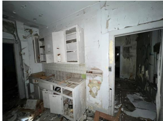
Picture 32: View of the Kitchen area on the ground level of the Old heritage Home, facing southwest.
