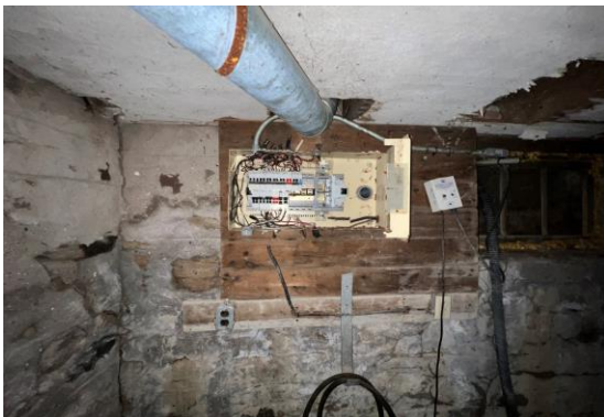
Picture 29: View of the disconnected electrical panel in the basement of the Old Heritage Home, facing northeast.
