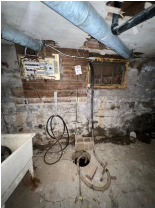
Picture 31: View of broken sump pump right next to the disconnected electrical panel in the basement of the Old Heritage home, facing northeast.
