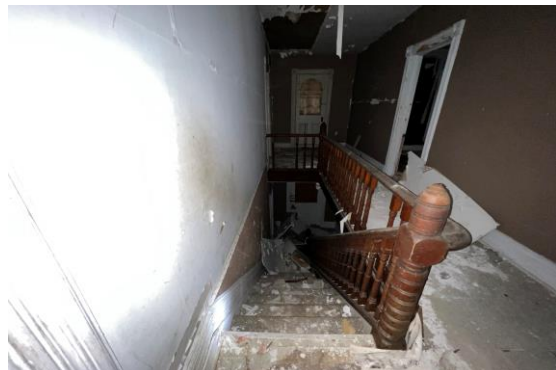
Picture 36: View of the staircase leading main floor from the upper level of the Old Heritage home, facing west
