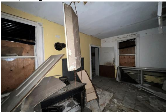
Picture 41: View of the dining area connecting to the extended garage of the Old Heritage home, facing southwest.
