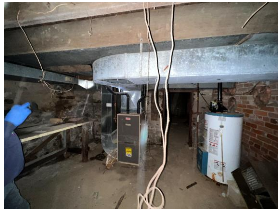
Picture 28: View of the Furnace in the basement of the Old Heritage Home, facing northeast.
