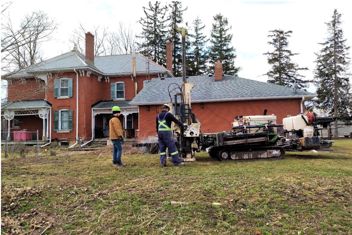
Photograph No. 3 – View of the advancement of borehole BH121-22 south of the farmhouse in the vicinity of the former in-ground pool.
