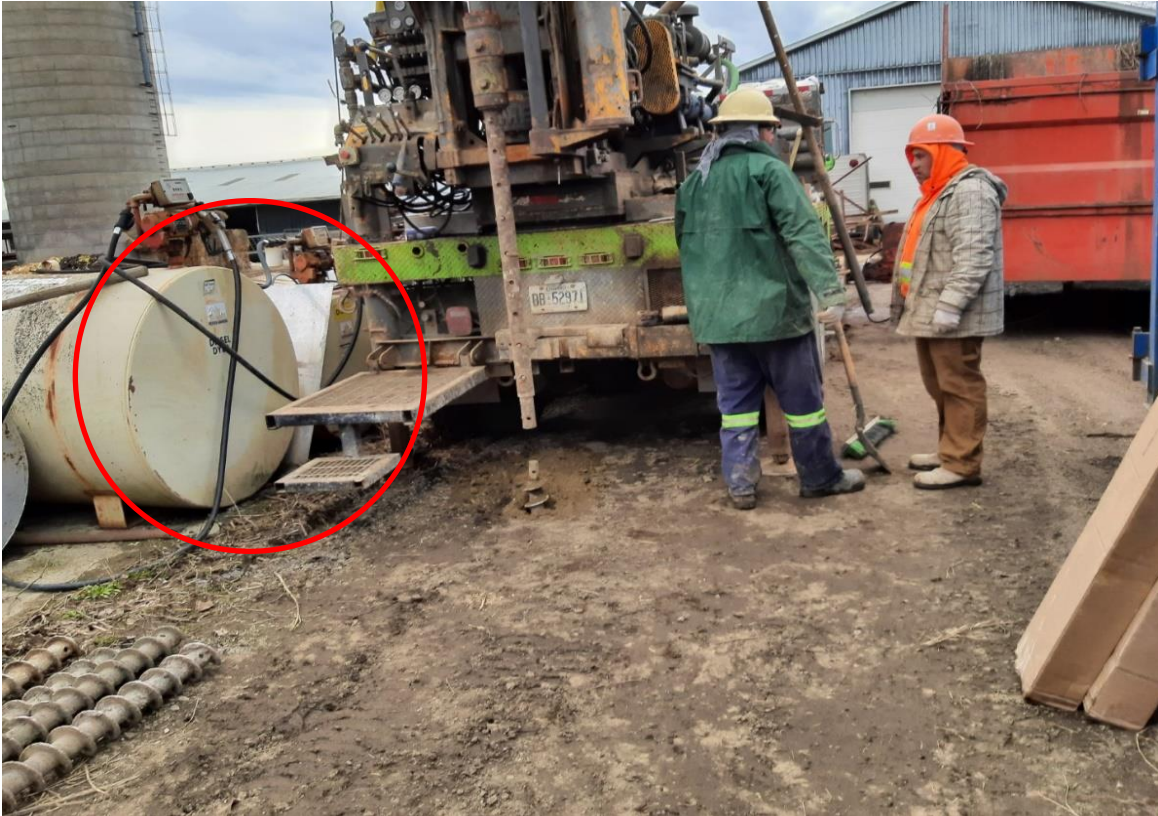
Photograph No. 7 – View of the advancement of borehole MW123-22 in the vicinity of the diesel ASTs.
