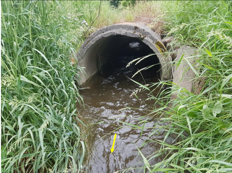
A degraded tractor crossing was present within the reach. The concrete culvert was separated through the middle and flows were undermining the feature.
