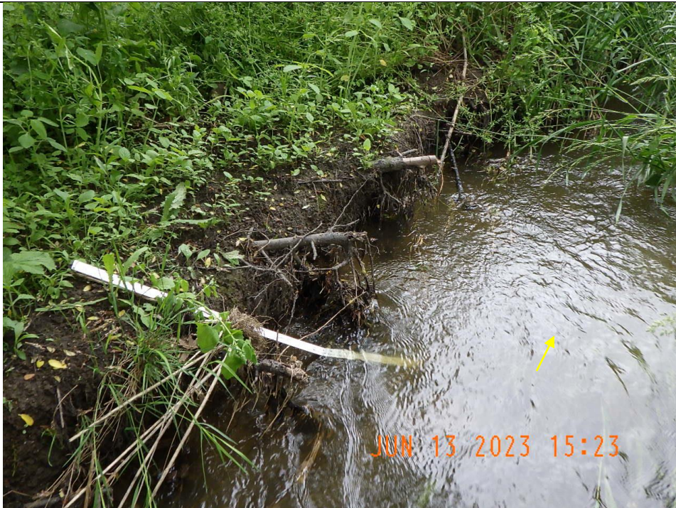
Bank erosion was observed through 30% to 60% of the reach. Undercuts, exposed tree roots, and fallen/leaning trees were observed indicating the channel is widening.
