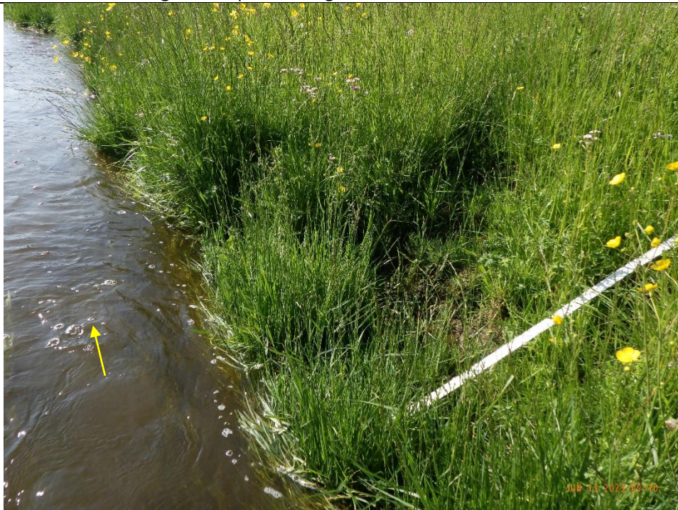
Bank slumps and undercutting were noted throughout the reach. Bank material was primarily silt, sand, and some clay.
