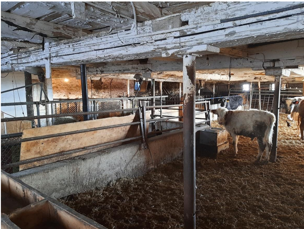
Photograph No. 8 – Interior view of the lower level of the two-storey barn.
