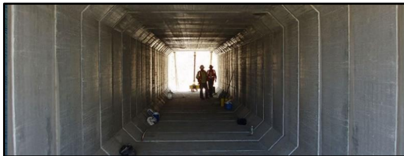
Image 1 – Manned StormCrete access
