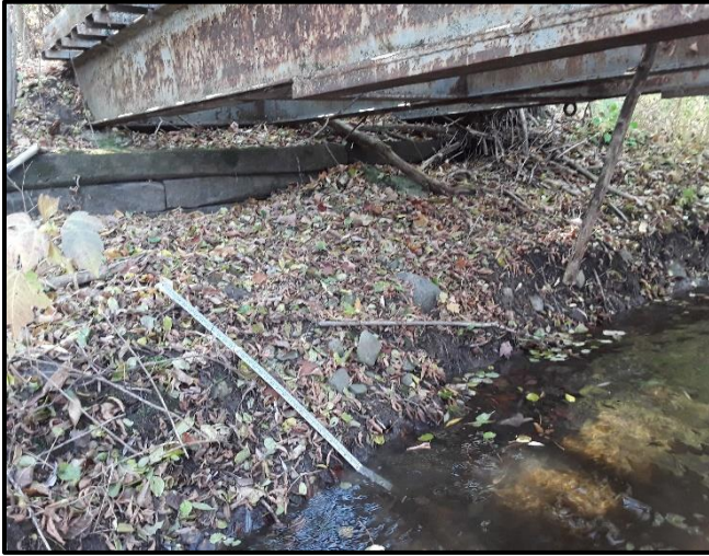
Photograph 13. Location 12. Reach WHT-1 West Humber River Tributary. Upstream view of right bank under pedestrian bridge. Bridge footings exposed. View: US Date Taken: November 8, 2022 Site: 12522 & 12306 Torbram Rd, Caledon ON
