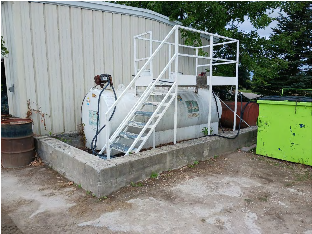
Photo H7 (South): 2000L AST compartmentalized to hold both gasoline and diesel in maintenance yard. Second smaller AST behind 2000L tank is no longer in use.
