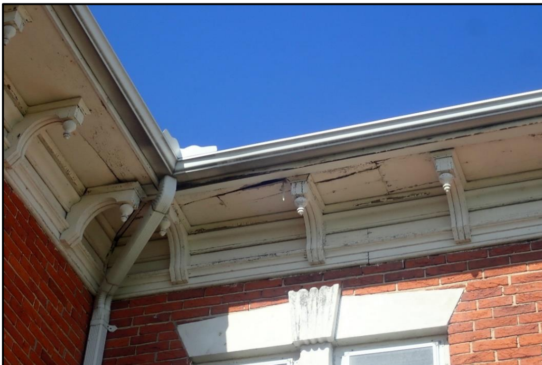
Photograph 3. Potential Bat Maternity Roosting Habitat: Cracks in the Soffit of the Residential Home (April 7, 2021)
