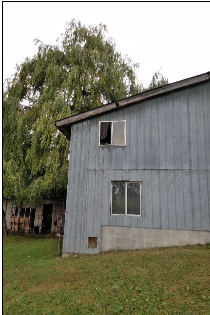
Photograph 4. Potential Bat Maternity Roosting Habitat: Multiple Gaps in Roof (September 12, 2023)
