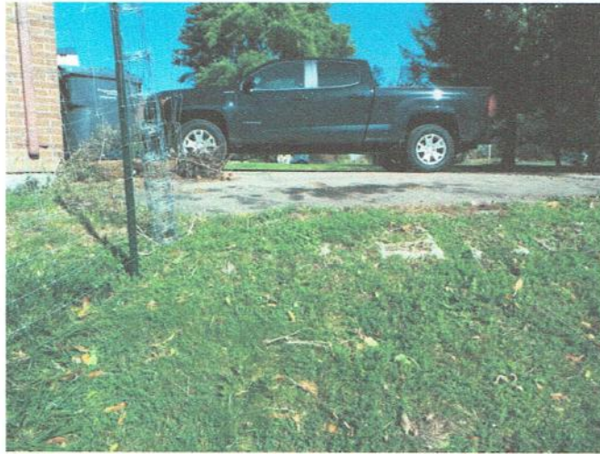
Photo No. 4: Buried Concrete Block Foundation northwest corner of the Residential Dwelling
