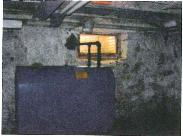
2. View of the fuel oil AST located in the basement facing north.
