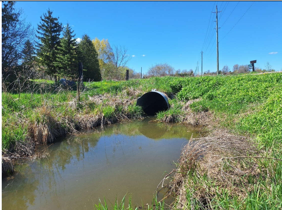
A scour pool was present downstream of the culvert at the upstream reach break.
