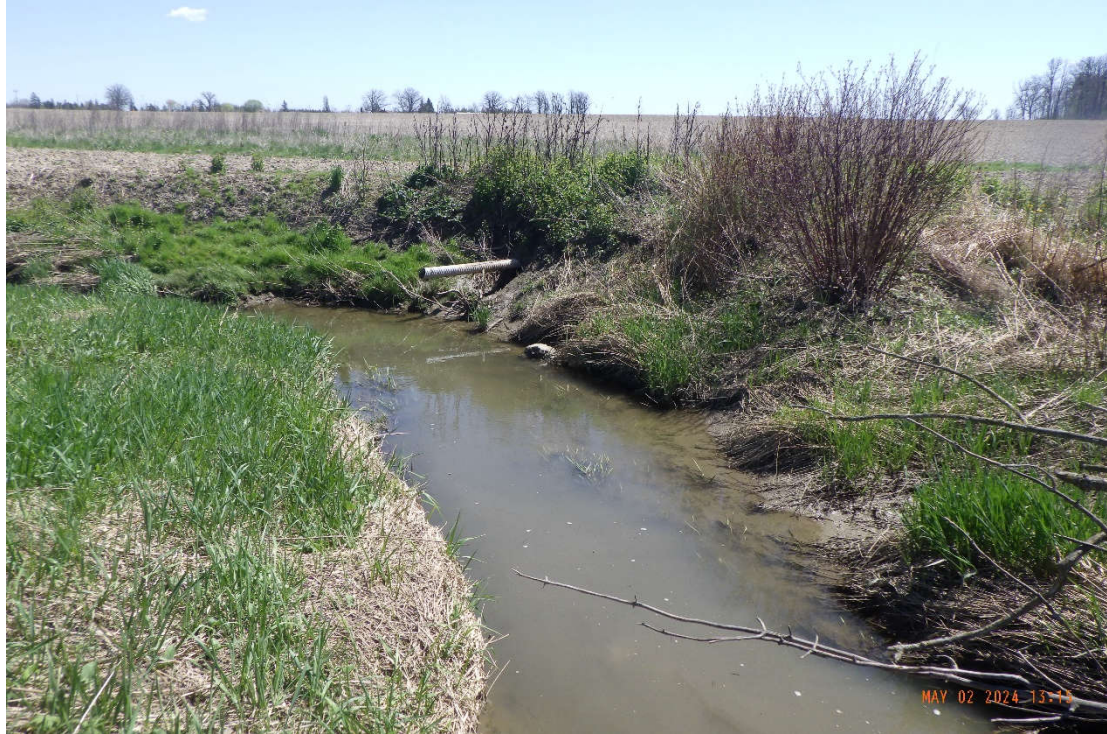
An exposed tile drain that was previously buried was observed at an outer bank of a meander bend and was in poor condition.
