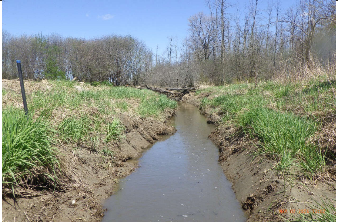
One localized area in the downstream portion of the reach showed evidence of recent dredging (sloped bare banks).
