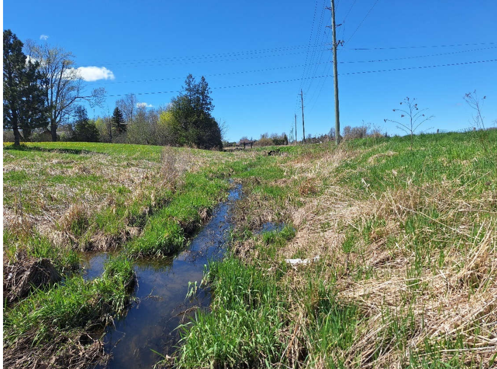
Multiple flow paths were observed in some locations.
