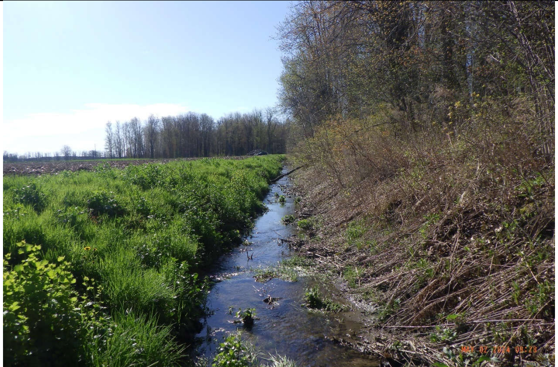
The reach was a straight channel with moderate entrenchment and lacked bar forms.
