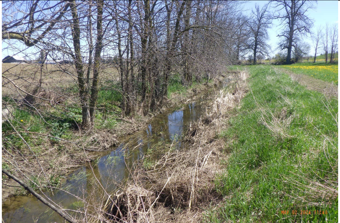
In the upstream portion of the reach a localized row of trees was present along the banks, some of which were leaning or had fallen into the channel.
