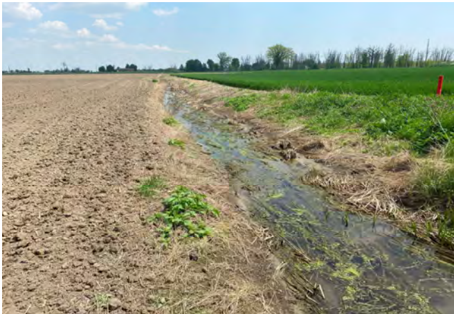
Photograph 15: Alloa Drain, looking downstream from Fraser Drain confluence – upstream segment of feature (May 15-16, 2024).
