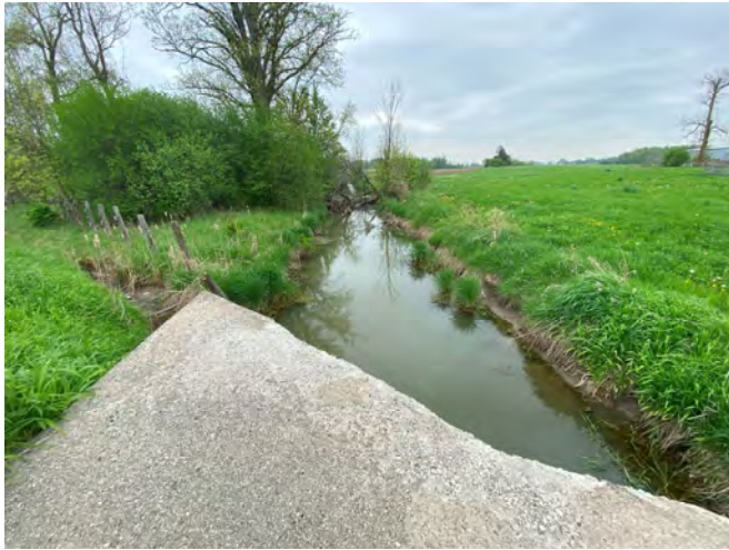
Photograph 13: Alloa Drain, looking upstream (southwest) from culvert inlet at Chinguacousy Road (May 15-16, 2024).
