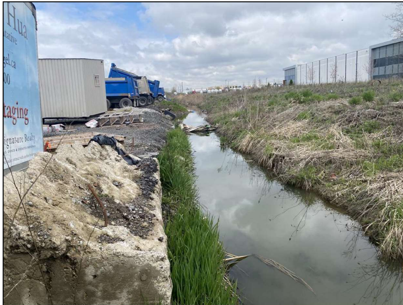
Photo 1. Concrete, fill and truck parking along the top of the west bank (photo taken facing upstream, north).
