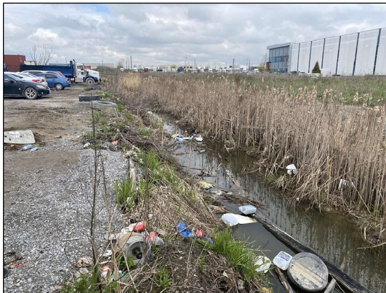
Photo 2. Fill and garbage along west bank, dense vegetation in the channel along east bank (photo taken facing upstream, north).
