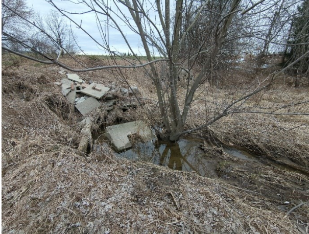
Photo 9 – Upstream extent of uncovered portion of Reach WHT4(3)4-2, downstream of piped portion.
