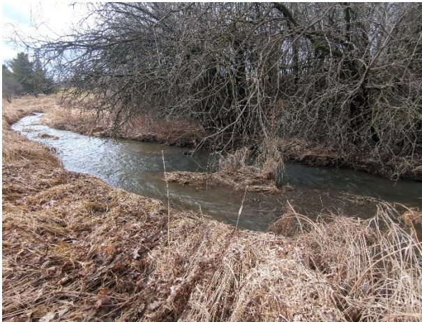
Photo 19 – Reach WHT4(3)2-1 traverses Mayfield Golf Course. Significant basal scour was observed throughout.
