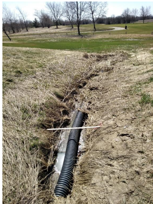
Photograph 13. HDF 4A – Downstream View of Tile Drain (April 12, 2023).
