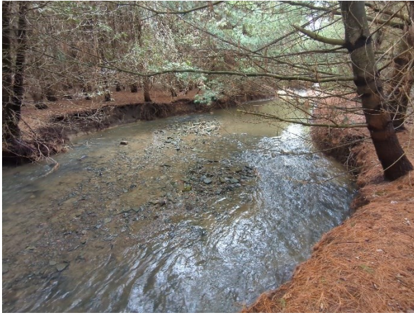
Photo 13 – Downstream portion of Reach WHT4(3)3-1, downstream of culvert. Watercourse displays severe degradation / widening.
