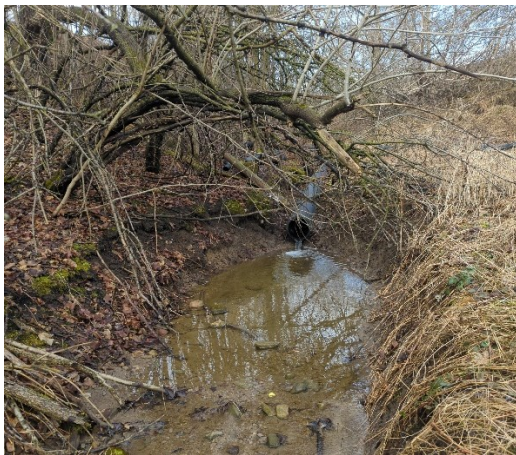
Photo 3 – Scour pool at downstream extent of pipe, in Reach WHT4(3)6-1.
