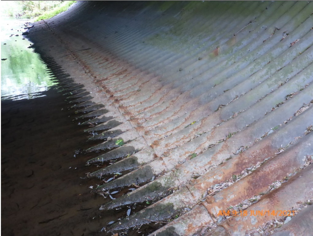
Coatings - Structural Steel - Light to Severe Breakdown of Coating - Photo 21
