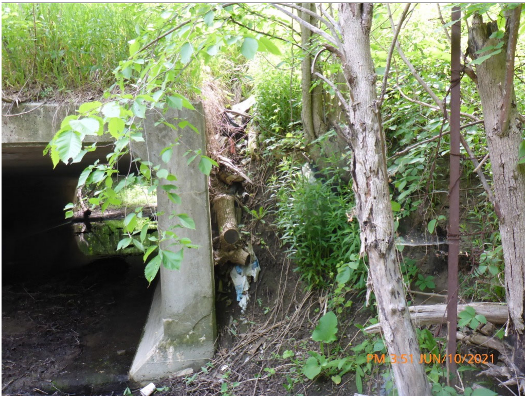
Embankments and Streams - Embankments - Severe Erosion - Northwest - Photo 20
