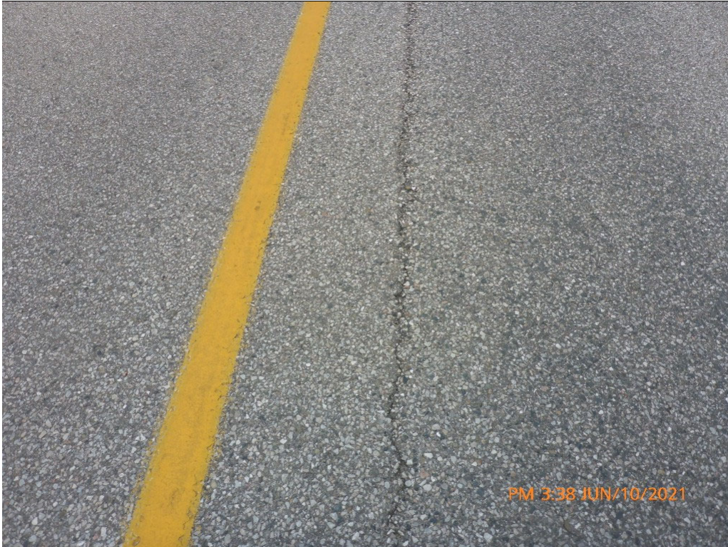
Approaches - Wearing Surface - Light Crack - Photo 5
