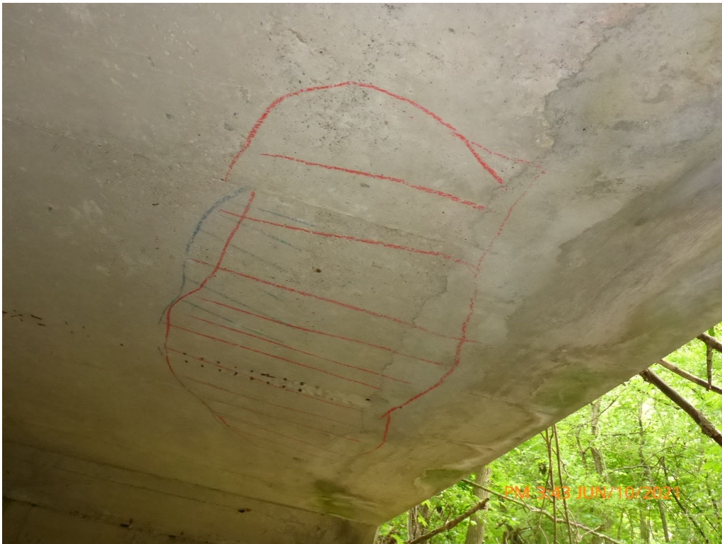
Culverts - Barrels - Severe Delamination on Soffit - Photo 12
