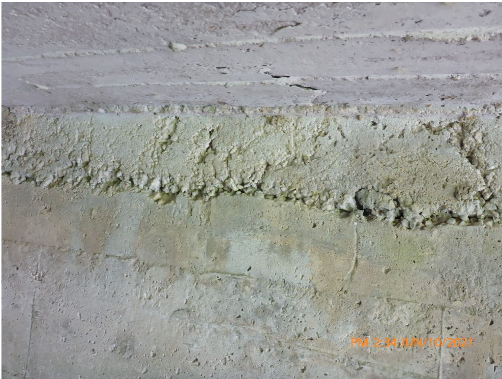
Abutments - Abutment Walls - Light to Severe Honeycombing - Photo 20
