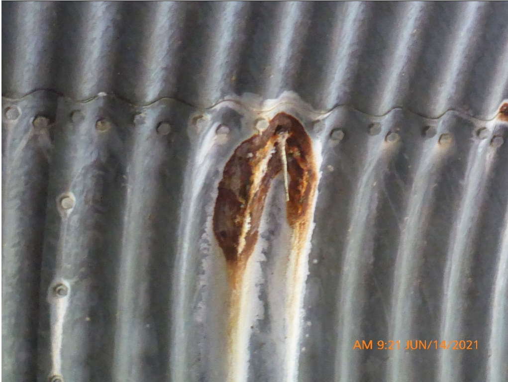
Culverts - Barrels - Stalactites on Wall - Photo 17
