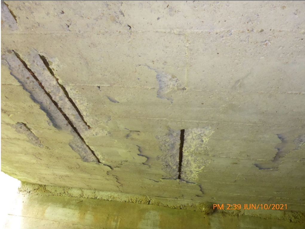
Decks - Soffit - Thick Slab - Interior - Severe Spalls - Photo 17
