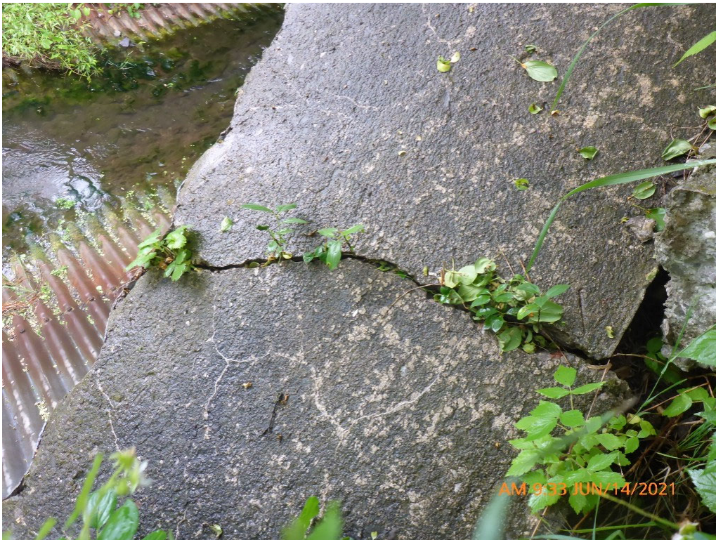
Culverts - Inlet Components - Wide Crack on Stiffener - SW - Photo 26
