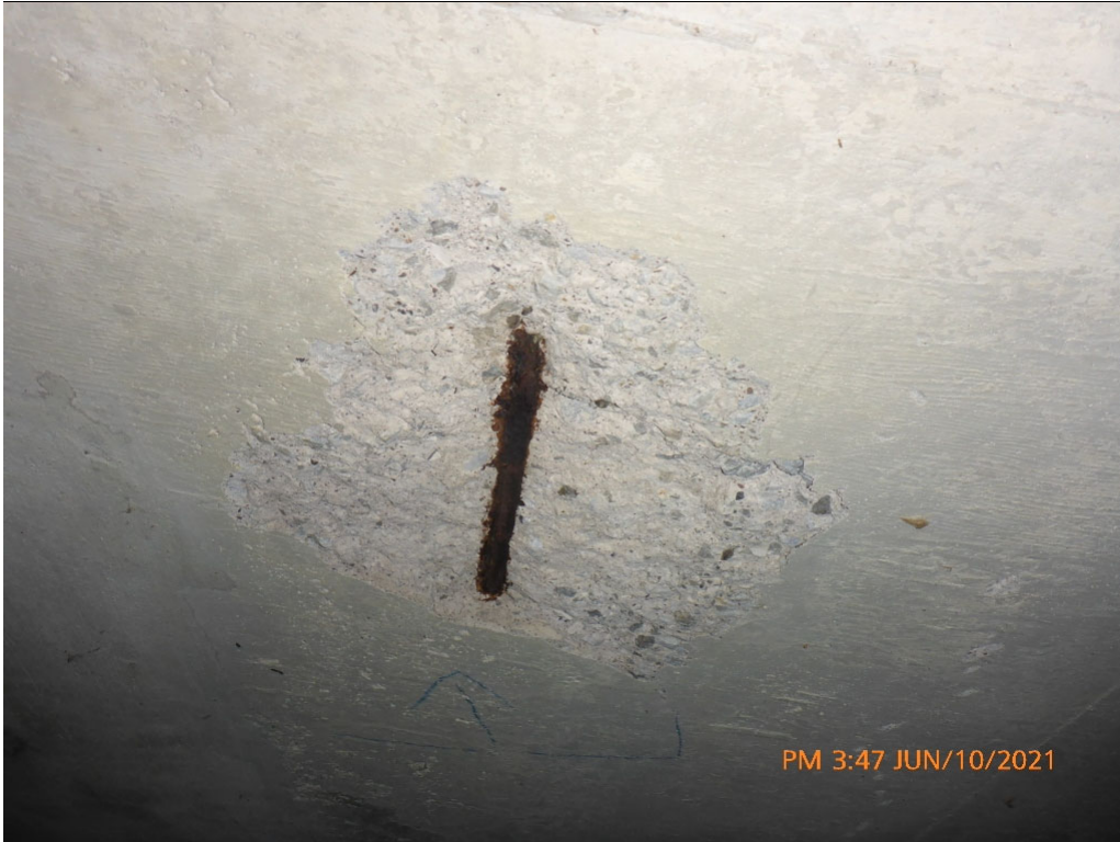
Culverts - Barrels - Severe Spall on Soffit - Photo 15
