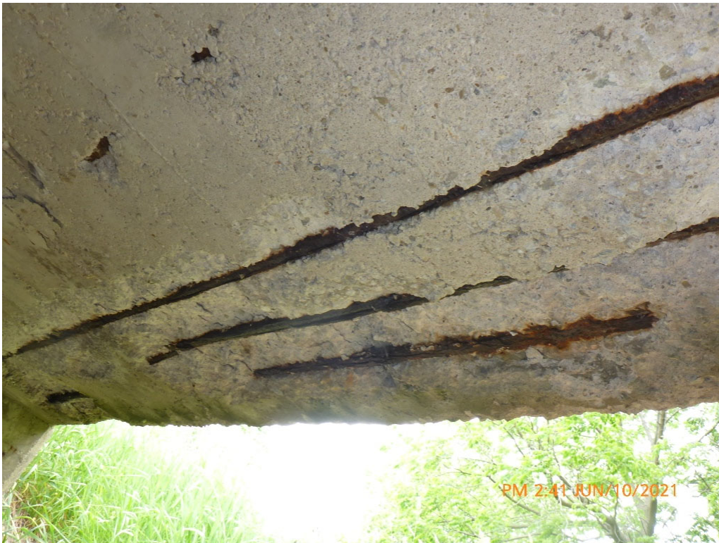
Decks - Soffit - Thick Slab - Exterior - Severe Spalls - North - Photo 12
