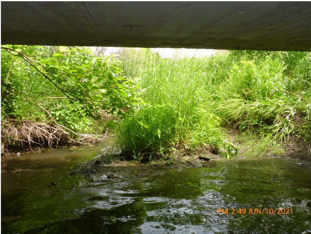
Embankments and Streams - Streams_Waterways - Aggradation of Watercourse - South - Photo 28
