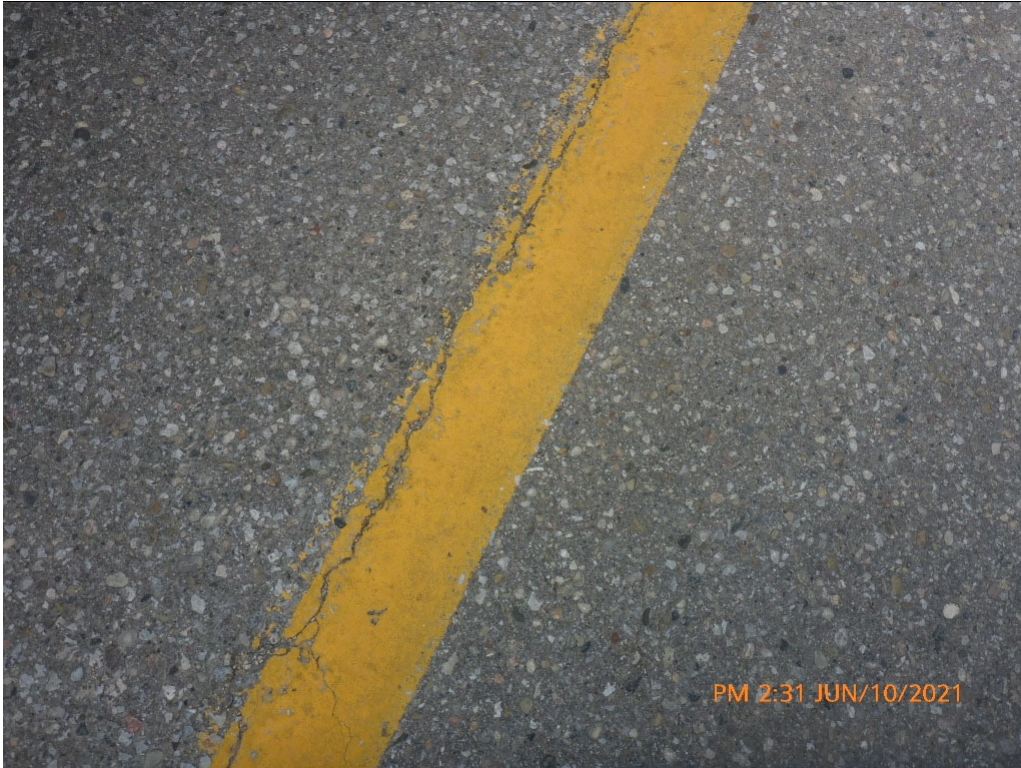
Decks - Wearing Surface - Light Crack - Photo 9
