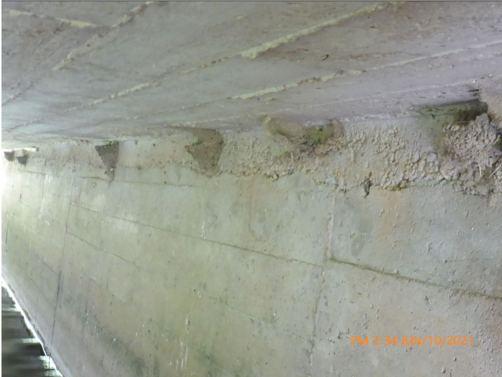
Abutments - Abutment Walls - Birds Nests - Photo 21
