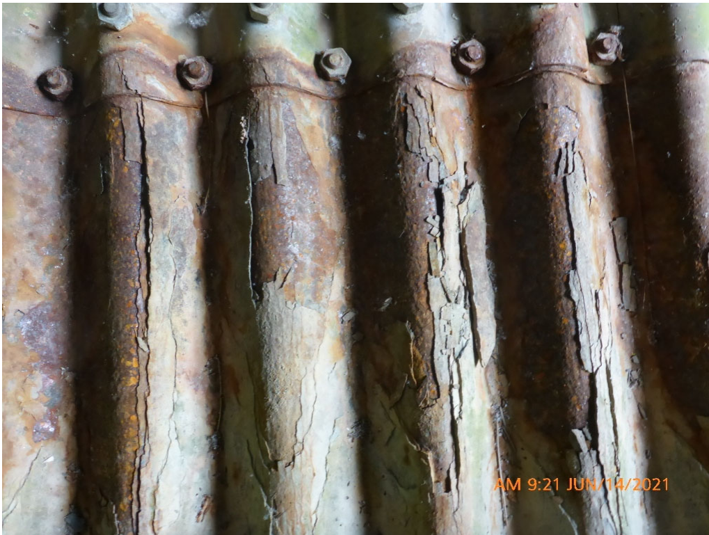
Culverts - Barrels - Medium Corrosion on Invert - Photo 16
