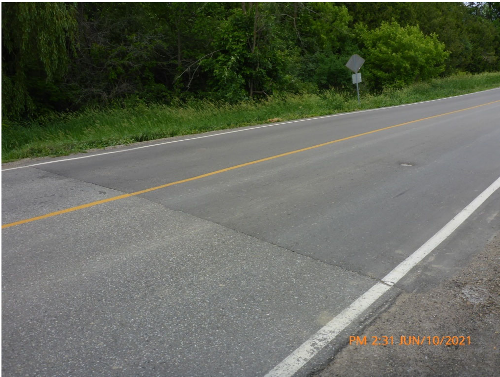
Approaches - Wearing Surface - East Approach Recently Resurfaced - Photo 8
