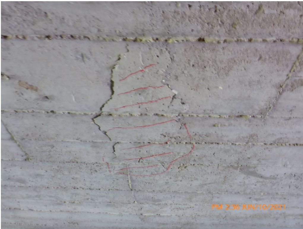
Decks - Soffit - Thick Slab - Interior - Medium Delamination - Photo 14
