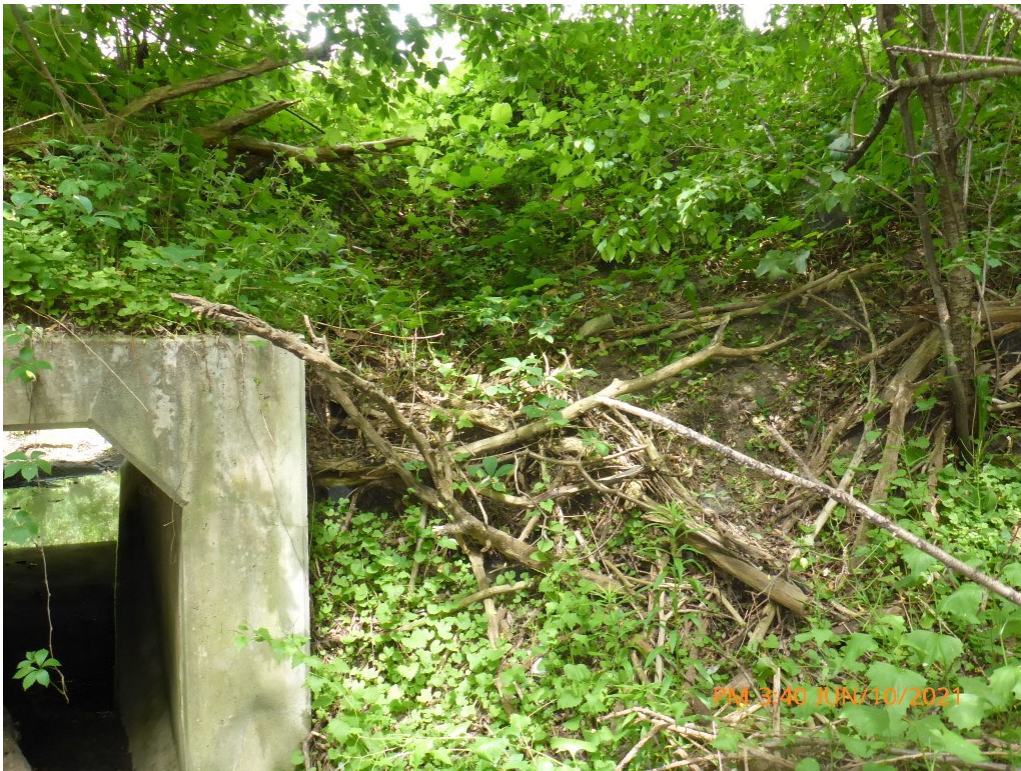
Embankments and Streams - Embankments - Medium Erosion - SW - Photo 18
