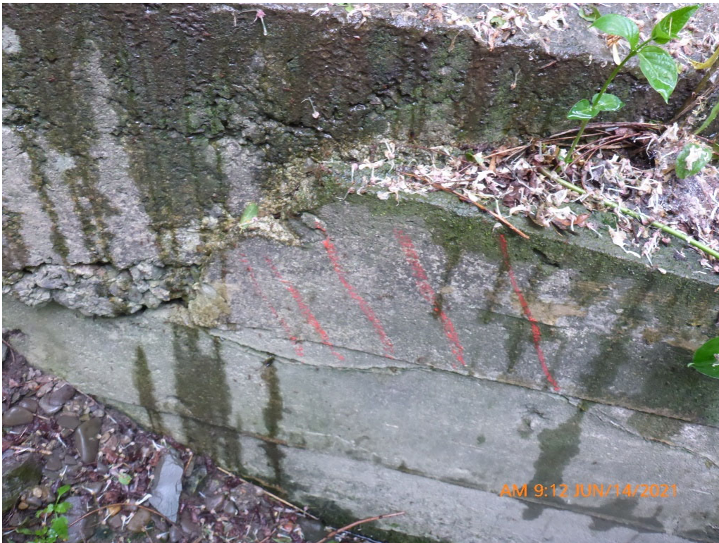
Culverts - Outlet Components - Light Delamination - SE Cut-off Wall - Photo 28
