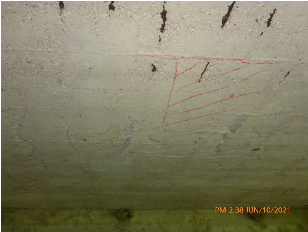
Decks - Soffit - Thick Slab - Interior - Severe Delaminations - Photo 16
