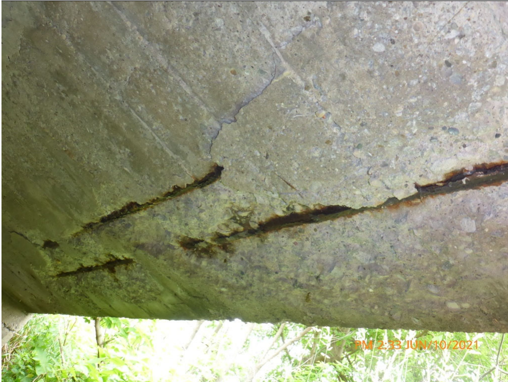
Decks - Soffit - Thick Slab - Exterior - Severe Spalls _ Delaminations - South - Photo 11
