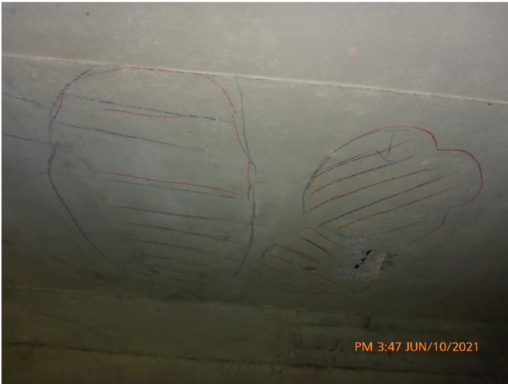
Culverts - Barrels - Severe Delaminations on Soffit - Photo 14
