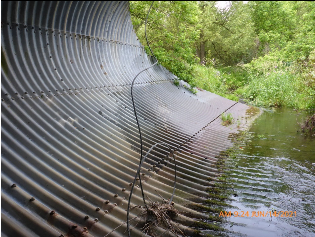
Culverts - Barrels - Cable Hanging into Barrel at West - Photo 19
