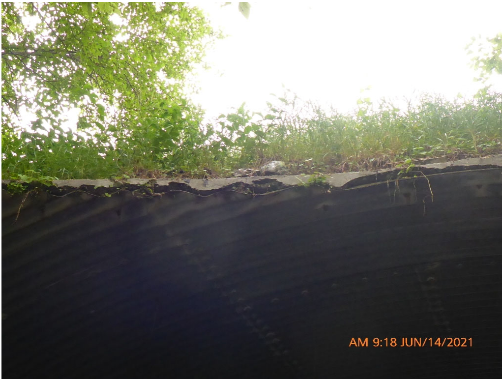
Culverts - Outlet Components - Light Spalls on Stiffener - Photo 34
