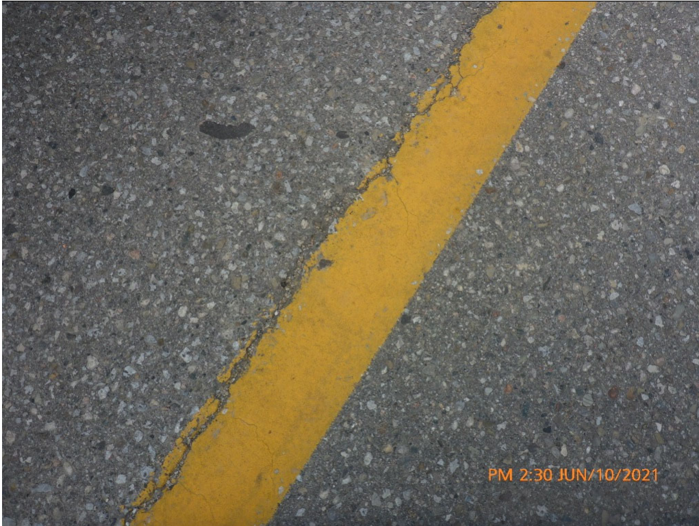
Approaches - Wearing Surface - Light Crack - West Approach - Photo 7
