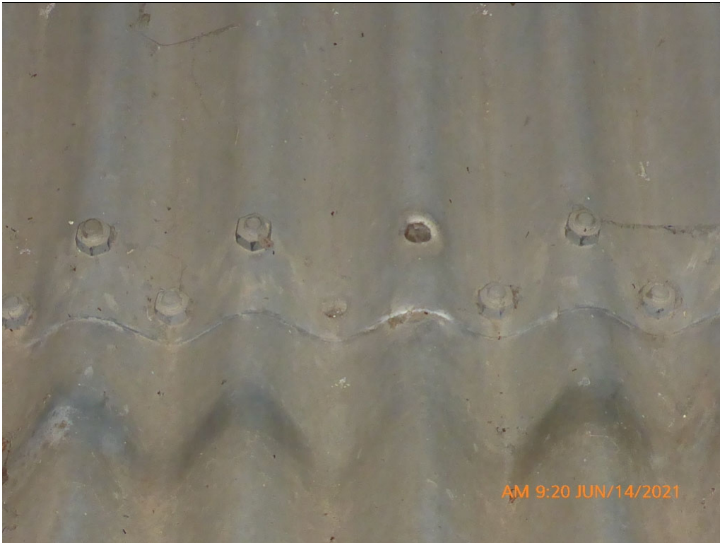
Culverts - Barrels - Missing Bolts - South Wall - Midspan - Photo 15
