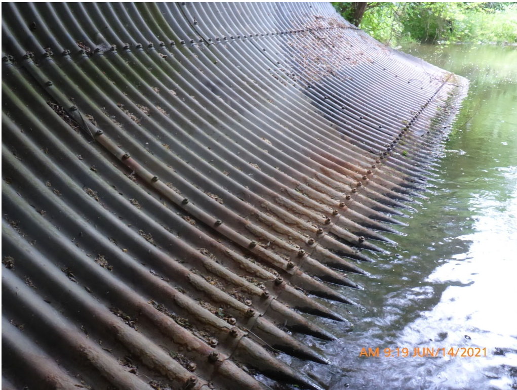
Culverts - Barrels - Overall Light Corrosion - Photo 14
