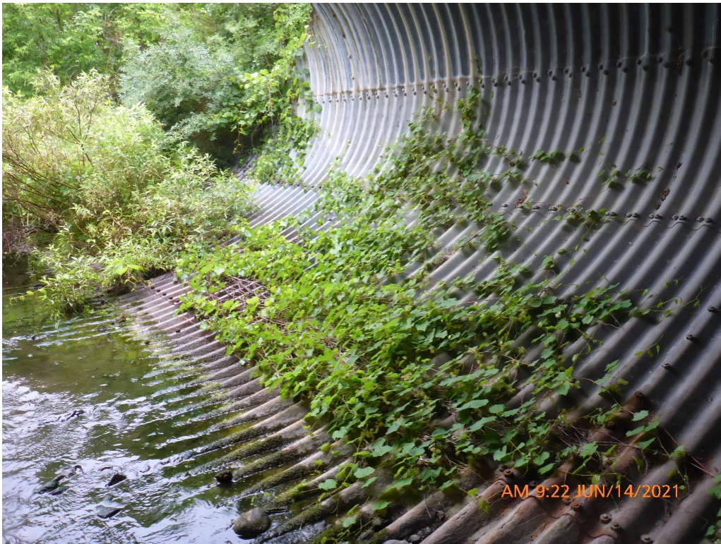
Culverts - Barrels - Vegetation Growing in Barrel - Photo 18
