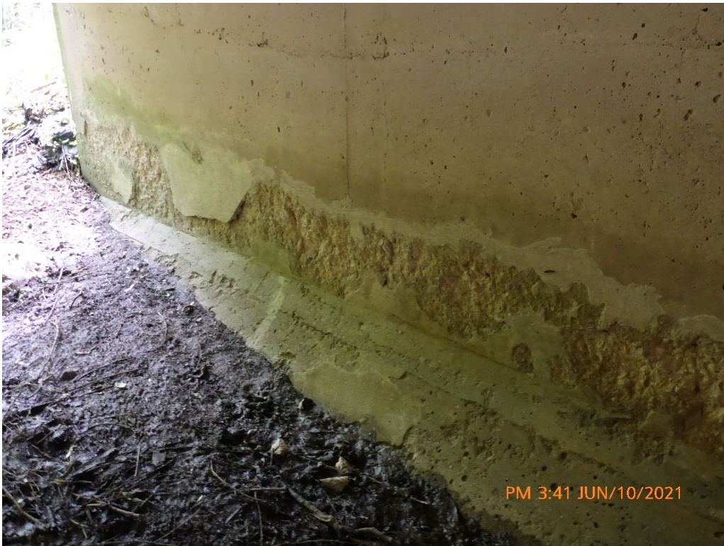
Culverts - Barrels - Severe Erosion on Wall - North Wall - Photo 10
