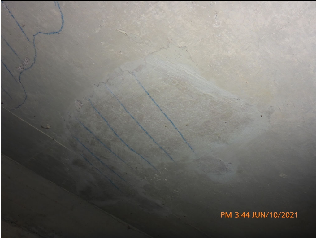
Culverts - Barrels - Debonded Concrete Patch on Soffit - Photo 13
