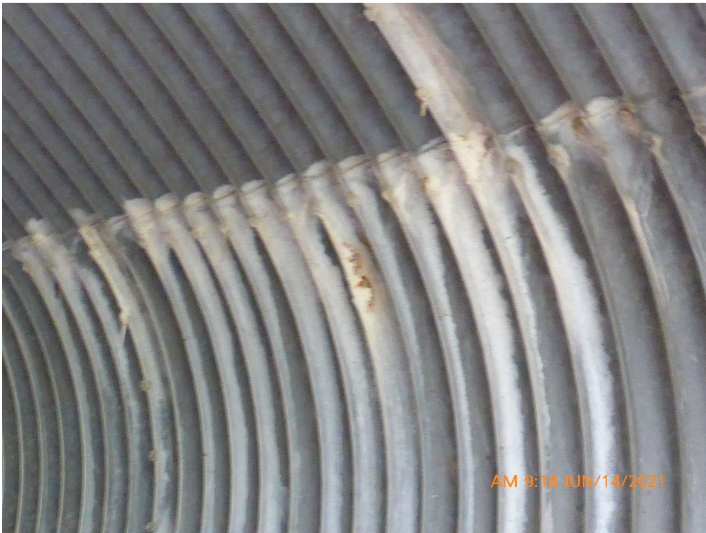
Culverts - Barrels - Efflorescence on Wall - Photo 12
