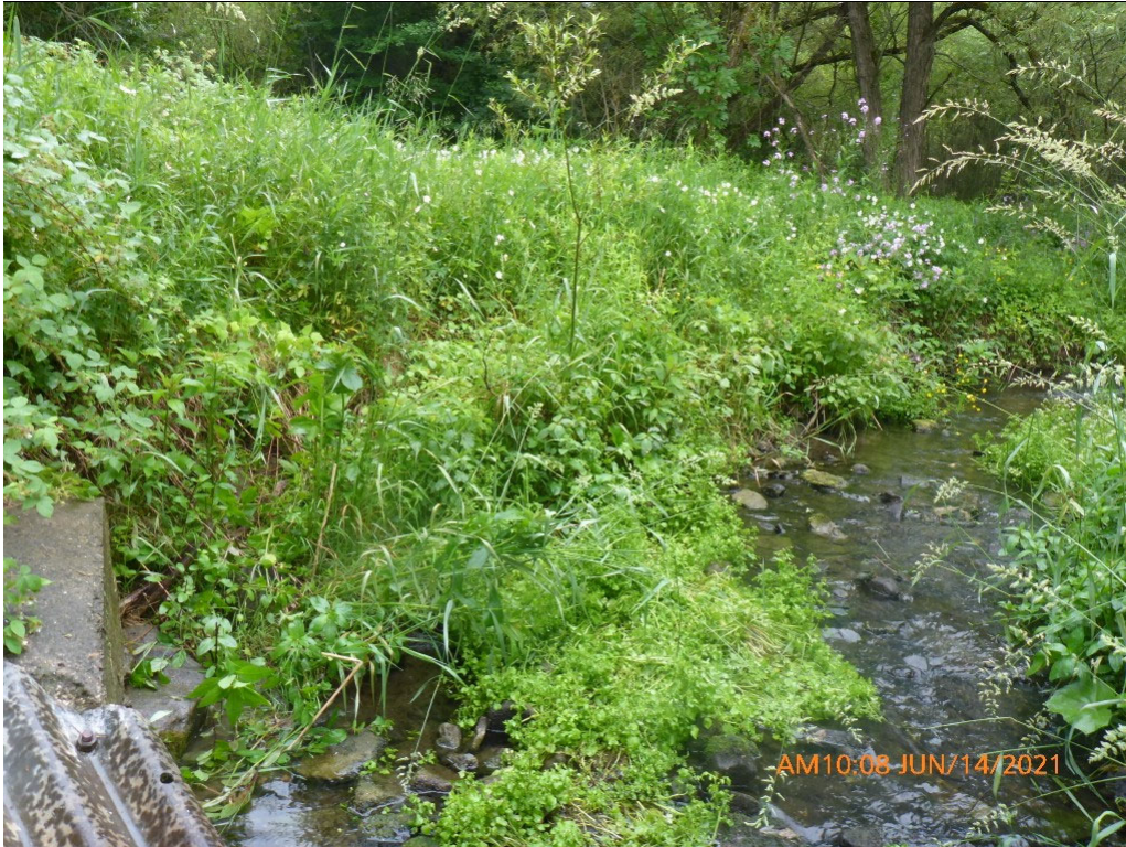
Embankments and Streams - Streams_Waterways - Medium Scour at SW - Photo 39
