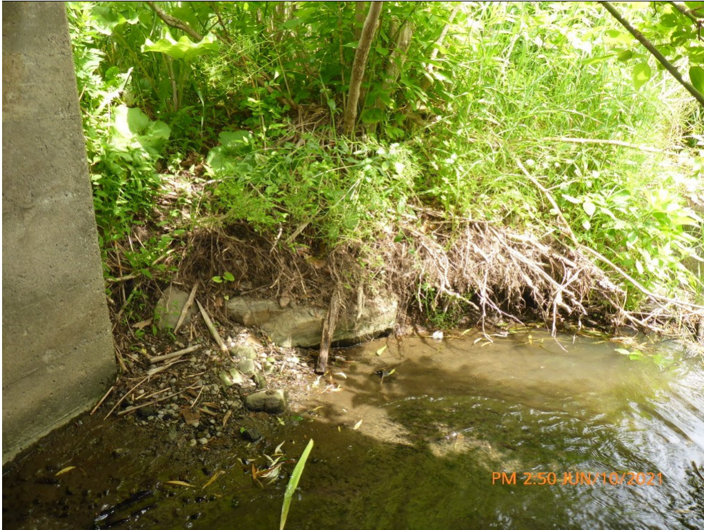
Embankments and Streams - Streams_Waterways - Light Scour - Southeast - Photo 27
