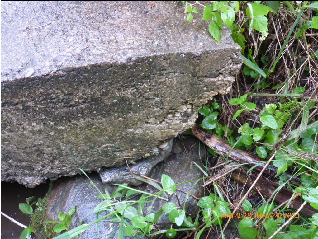
Culverts - Inlet Components - Severe Honeycombing on Cut-off Wall - SW - Photo 23
