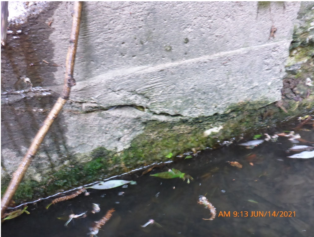
Culverts - Outlet Components - Wide Crack - NE Cut-off Wall - Photo 30
