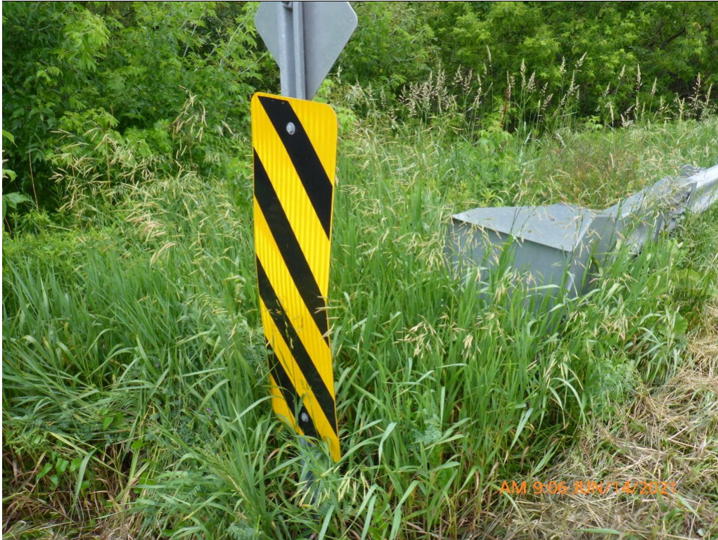
Accessories - Signs - Minor Damage to Southwest Hazard Marker - Photo 7
