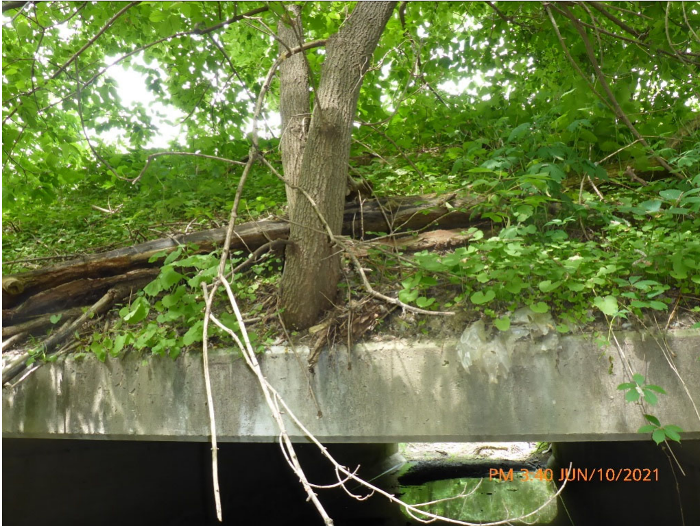
Embankments and Streams - Embankments - Tree Growing over Barrel - West - Photo 19
