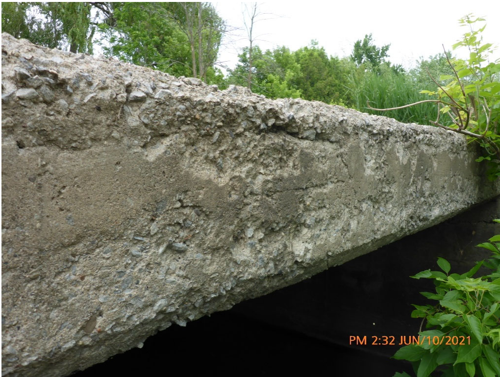
Decks - Soffit - Thick Slab - Exterior - Severe Scaling - South - Photo 10
