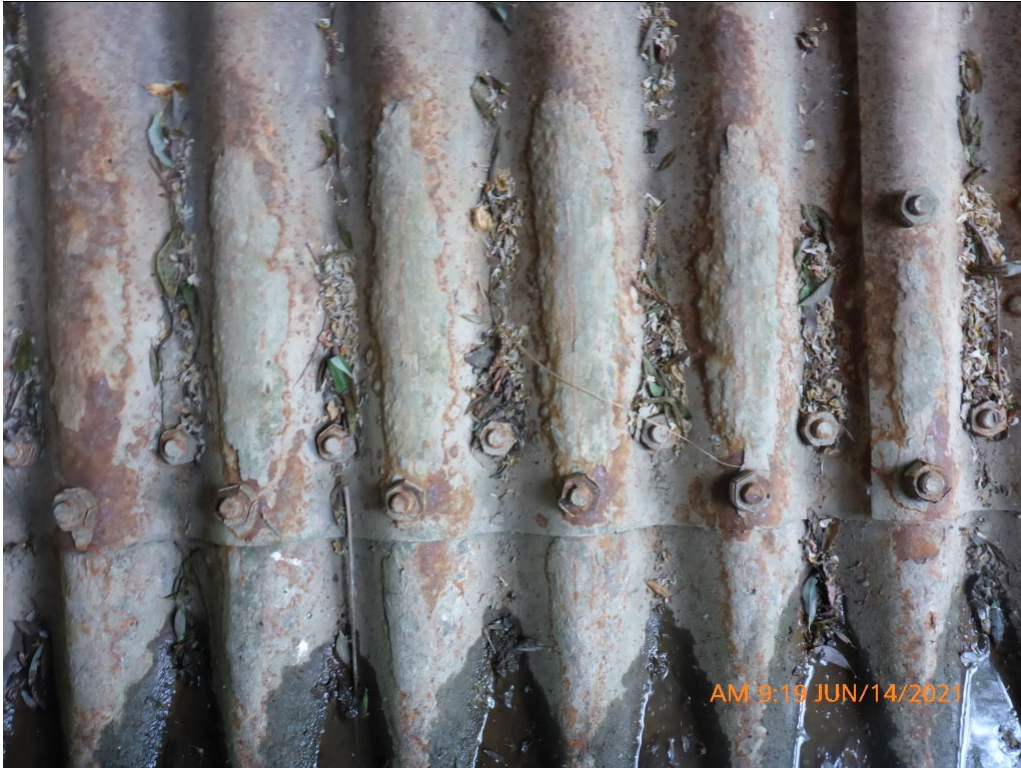
Culverts - Barrels - Medium Corrosion on Invert - Photo 13
