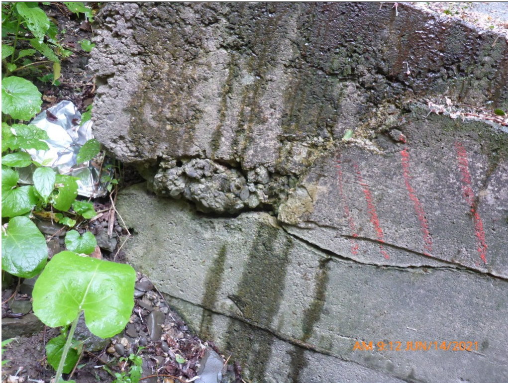
Culverts - Outlet Components - Severe Honeycombing - SE Cut-off Wall - Photo 29
