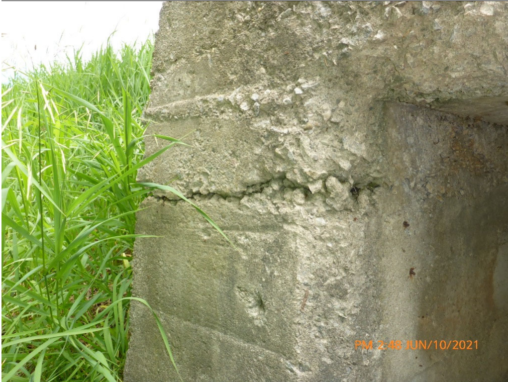
Abutments - Abutment Walls - Wide Gap at Cold Joint - Northeast - Photo 23
