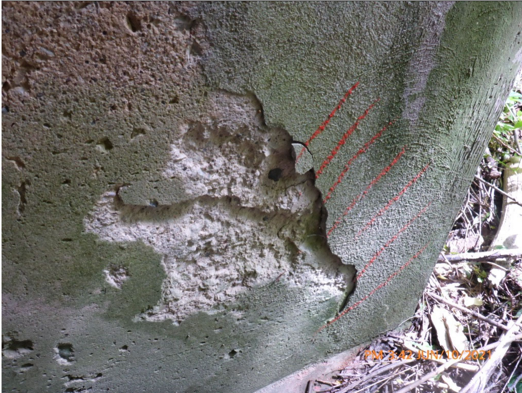
Culverts - Barrels - Debonded Concrete Patch - South Wall - Photo 11
