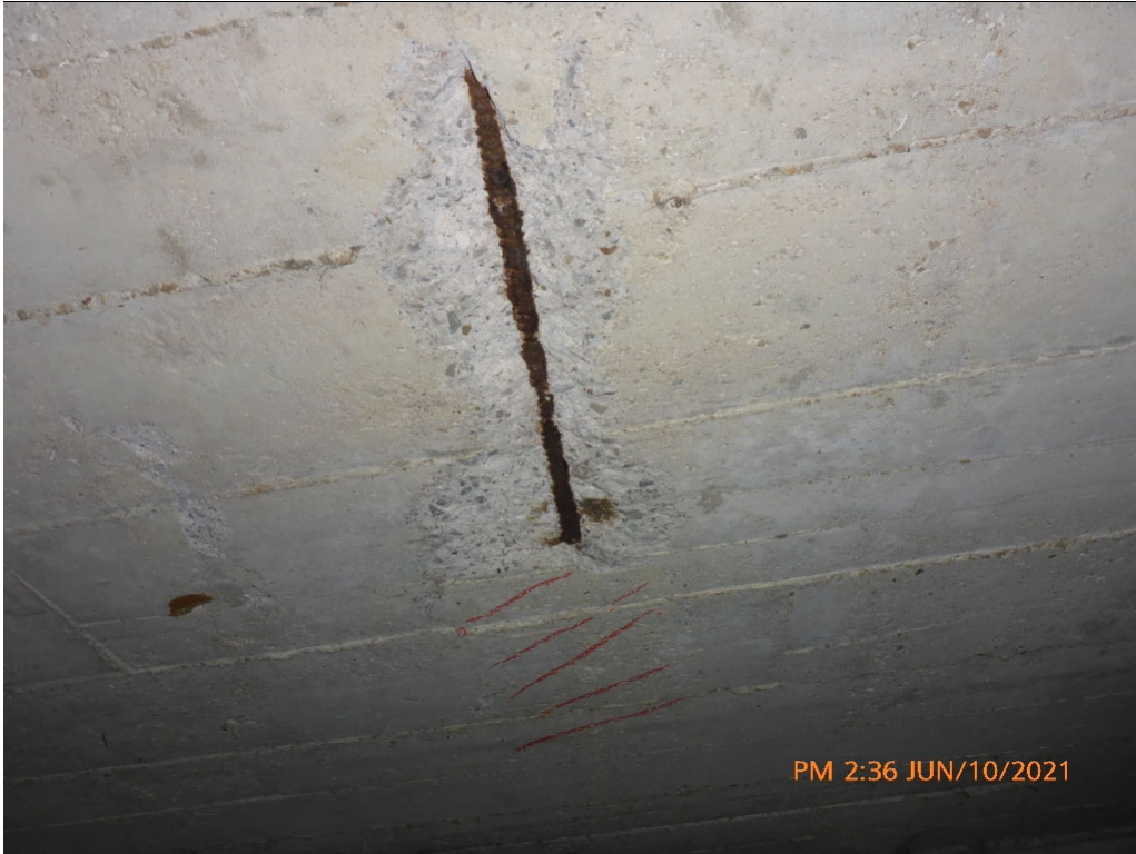
Decks - Soffit - Thick Slab - Interior - Severe Spall - Photo 15
