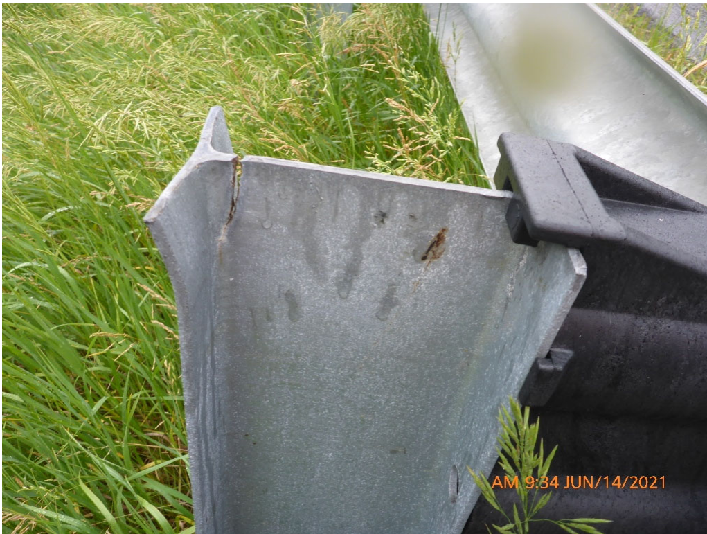
Approaches - Guide Rail - Crack in Post over Culvert at West - Photo 6
