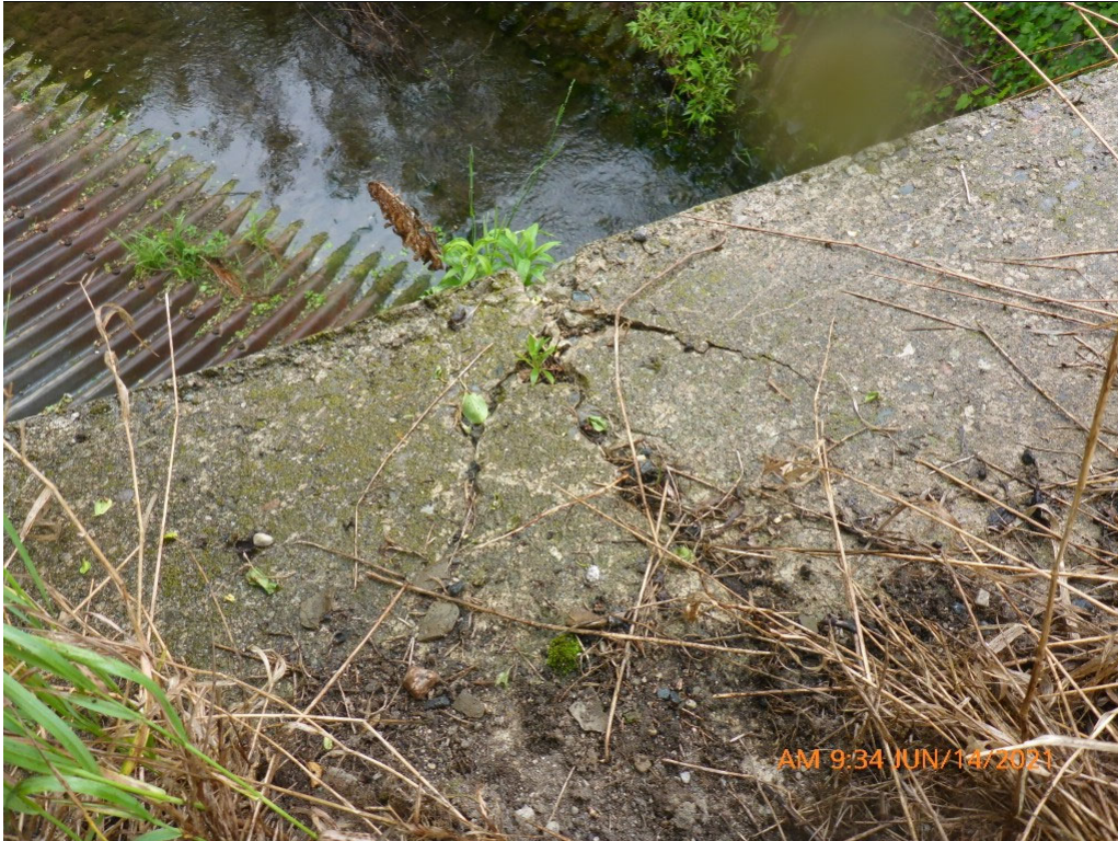
Culverts - Inlet Components - Wide Cracks on Stiffener - SW - Photo 27
