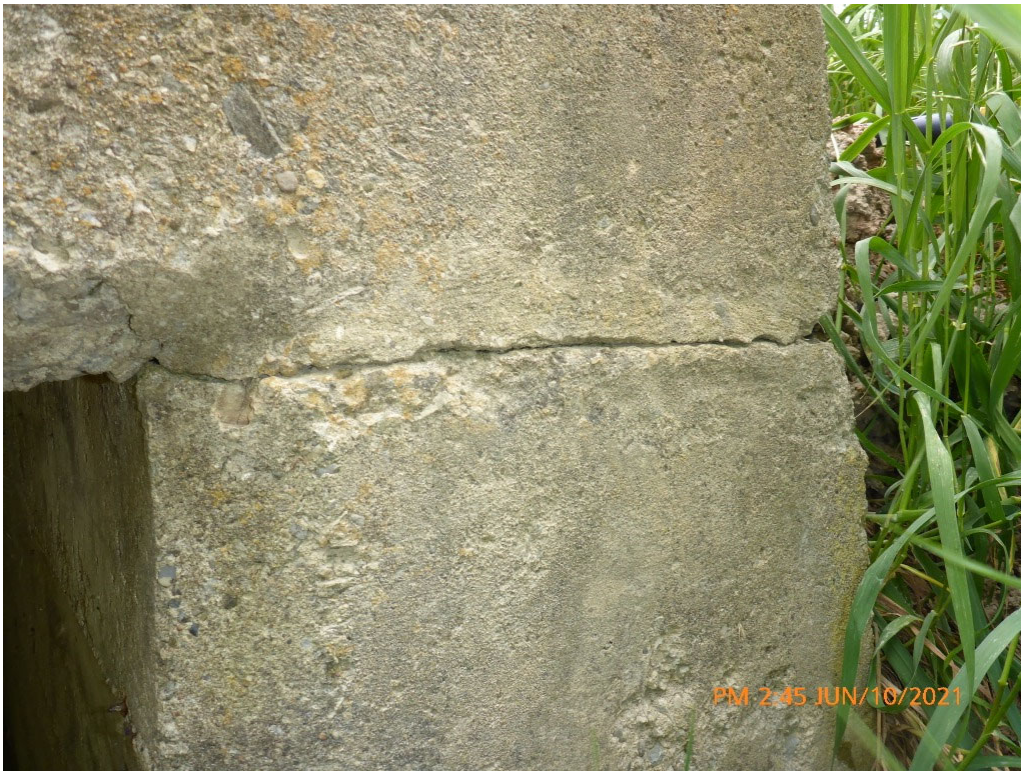
Abutments - Abutment Walls - Wide Gap at Cold Joint - Northwest - Photo 22
