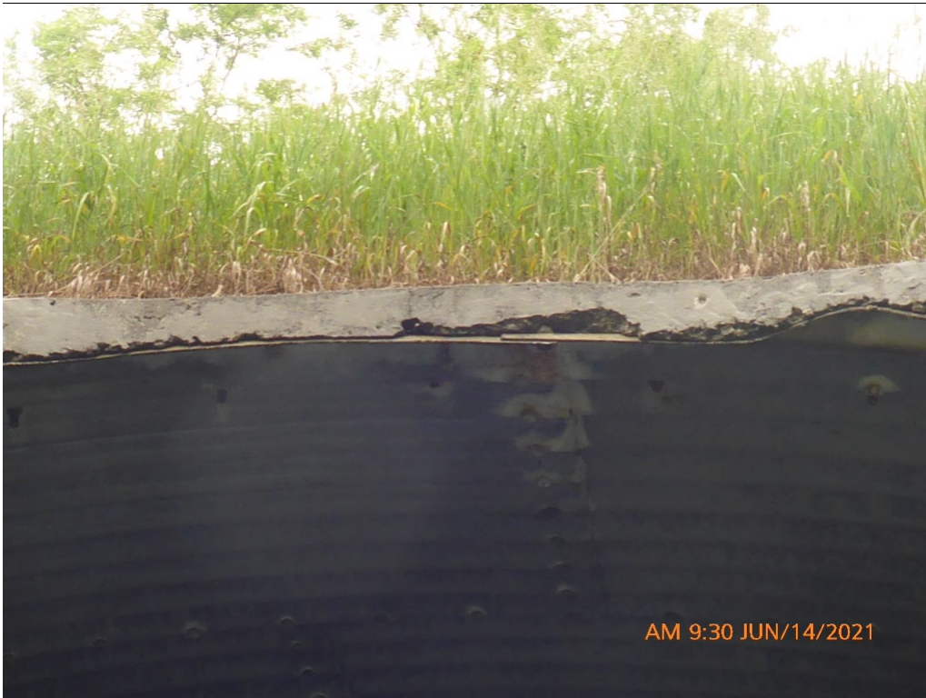
Culverts - Inlet Components - Light Spall on Stiffener - West - Photo 25
