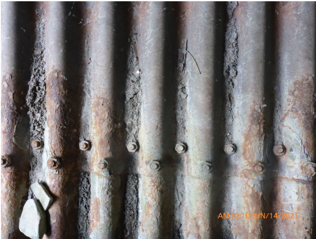
Culverts - Barrels - Improper Bolt Layout - Photo 20
