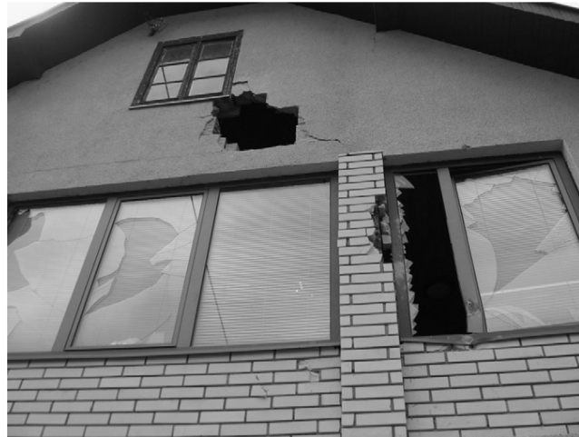
Fig. 9. The damage to structure (50 cm flyrock fragment at 320 m distance).
