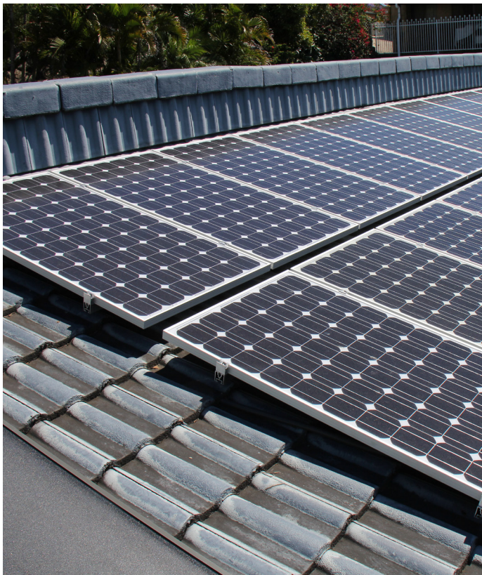
Figure 57: Rooftop Solar Panels
